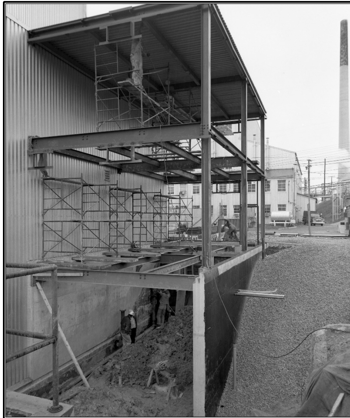
Figure A-38. Archival photograph showing the Change House addition to the north elevation of Building 3042 under construction, circa 1957 (ORNL Photo 42040).
