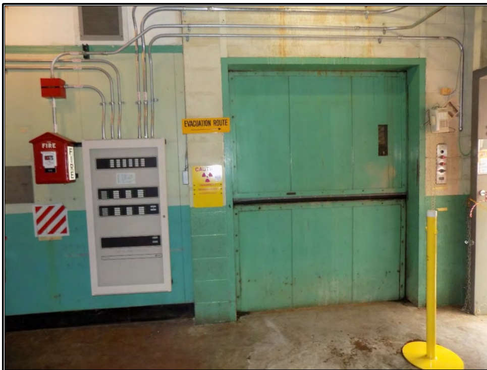
Figure A-24. Current photograph showing the elevator entry located in the southwest corner of Building 3042 at the second-level, facing south.
