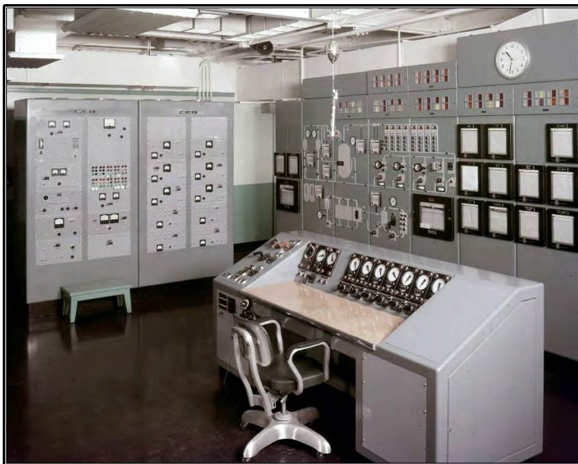
Figure A-42. Archival photograph showing the Control Room on the third floor of the north wing in Building 3042, circa 1958 (ORNL Photo 43209).
