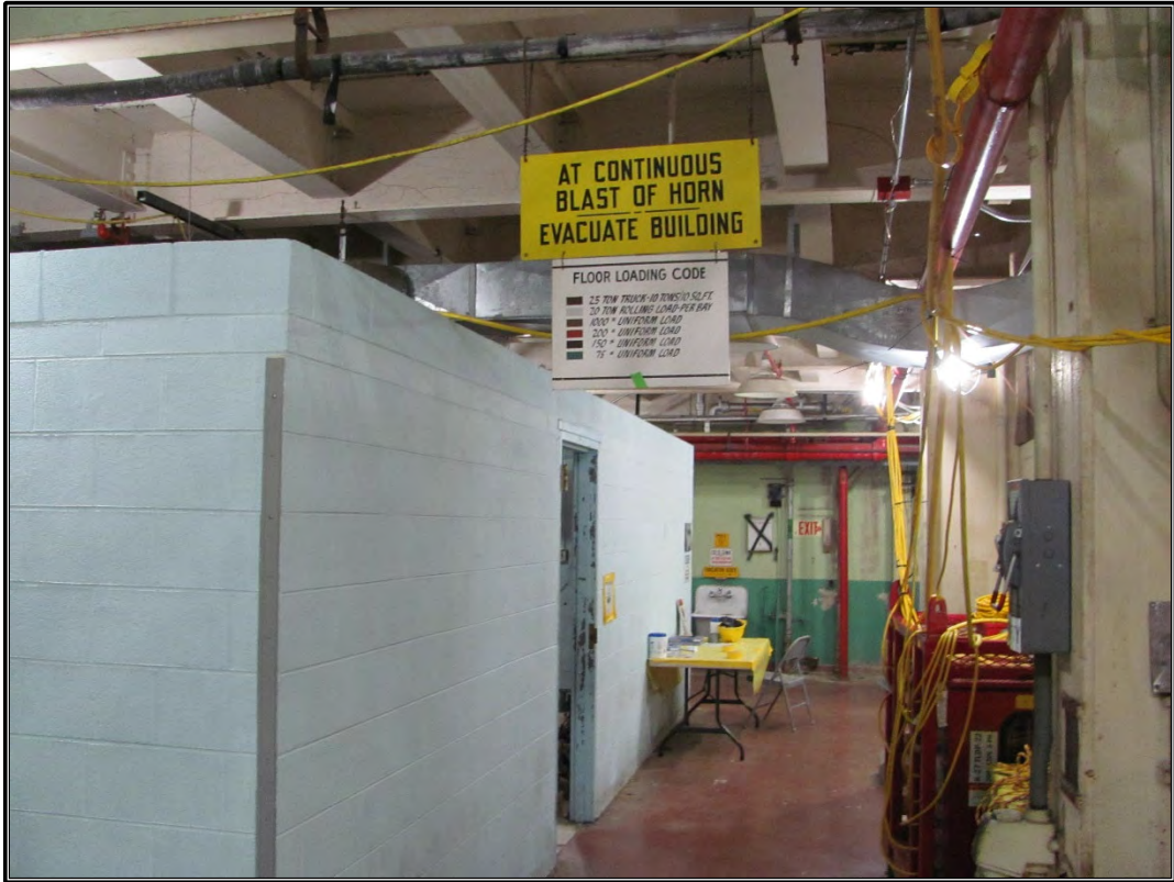
Figure A-21. Current photograph showing a portion of the first floor north corridor as well as the walls containing the Electrical Shop located on the north side of the ORR structure, facing west.
