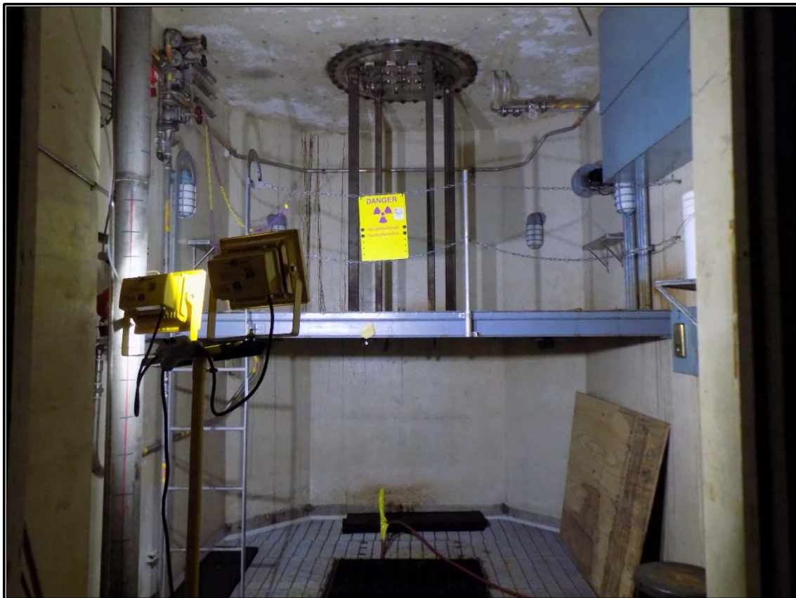
Figure A-10. Current photograph showing the ORR sub-pile room, or reactor pit, in the basement of Building 3042, facing west.
