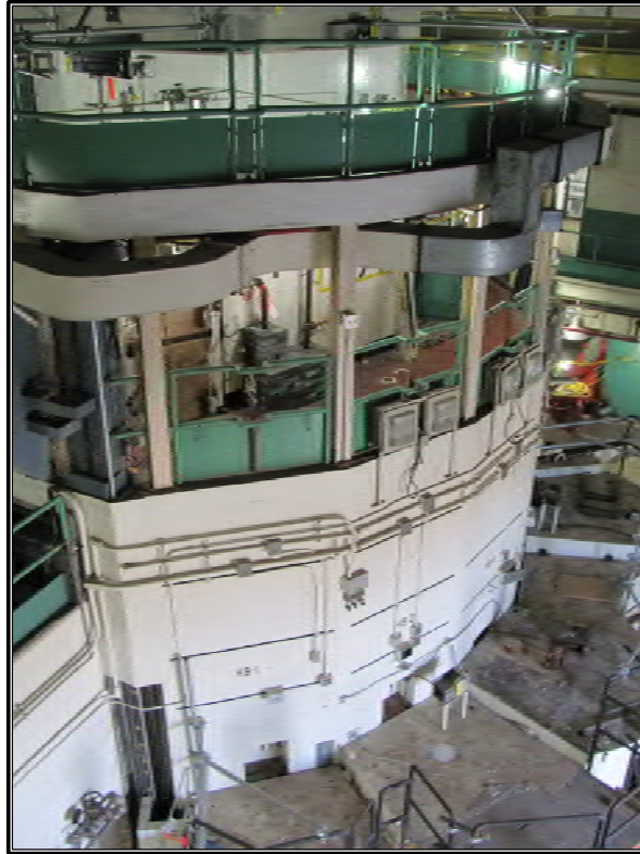
Figure A-13. Current photograph showing the east end of the ORR structure dominating the high bay of Building 3042 as seen from the second floor south corridor, facing north.
