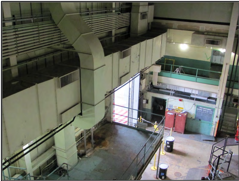
Figure A-16. Current photograph showing the east portion of the high bay in Building 3042, including the second-level platform on the east wall, as seen from the third floor north corridor, facing southeast.
