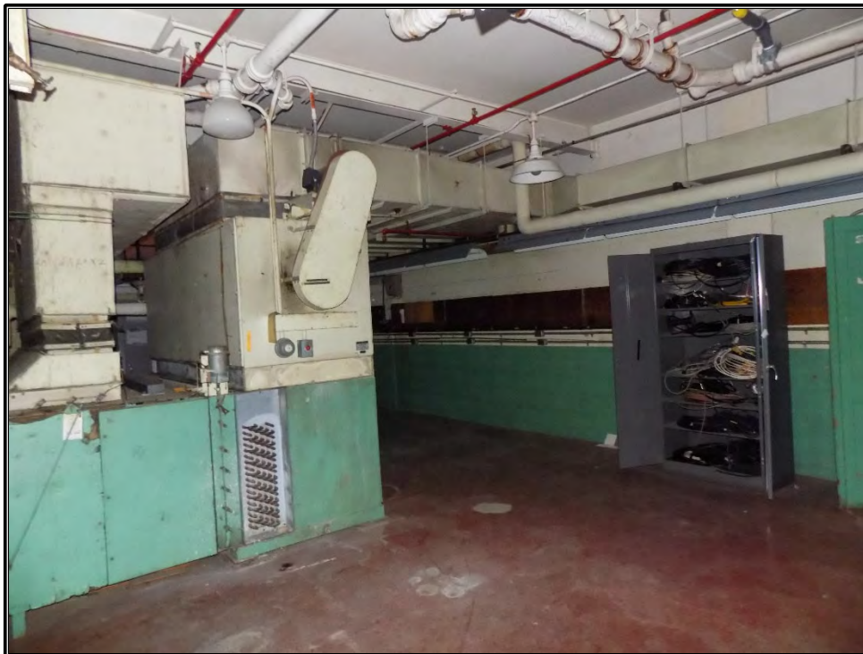
Figure A-20. Current photograph showing the Instrument Staff Shop area in the north wing of the first floor of Building 3042, including an air conditioning unit, facing southeast.
