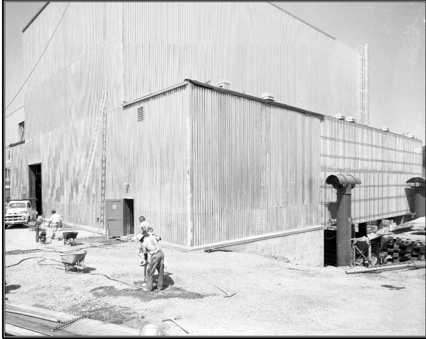
Figure A-37. Archival photograph, circa 1956, showing the west and south elevations of Building 3042 under construction, facing northeast (ORNL Photo 18606).
