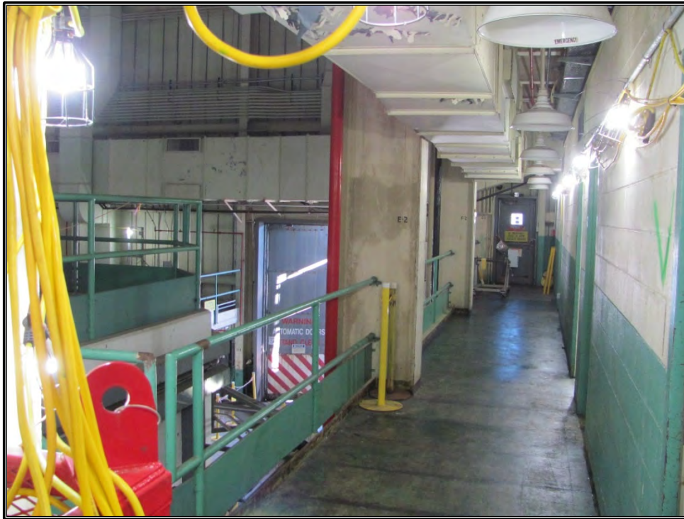
Figure A-25. Current photograph showing the second floor south corridor in the south wing of Building 3042, facing east.
