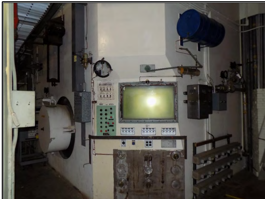
Figure A-18. Current photograph on the first floor of Building 3042 showing the containment cell, including the viewing window, located on the south side of the ORR structure, facing northwest.
