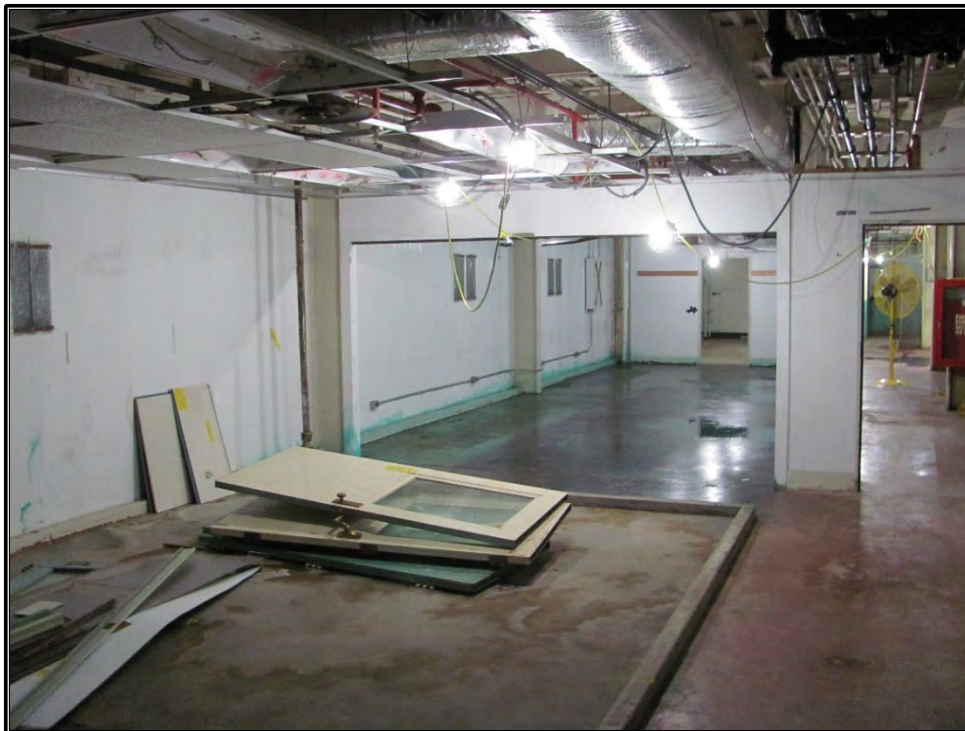
Figure A-30. Current photograph showing Room 308 on the third floor of the south wing of Building 3042, facing southwest.
