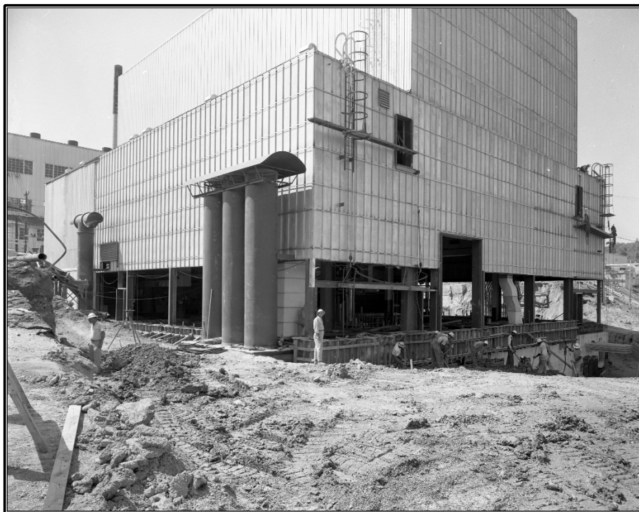
Figure A-36. Archival photograph, circa 1956, showing the south and east elevation of Building 3042 under construction, facing northwest (ORNL Photo 18608).
