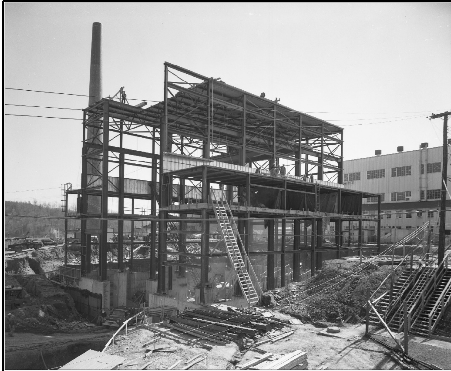
Figure A-35. Archival photograph, circa 1956, showing the steel framing in progress during the construction of Building 3042, facing southwest (ORNL Photo 17223).
