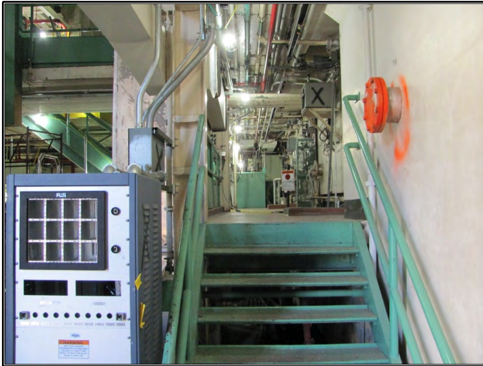
Figure A-23. Current photograph showing the stair access to the balcony of the ORR structure from the Truck Bay located on the second-level of Building 3042 at the west side of the ORR structure, facing east.
