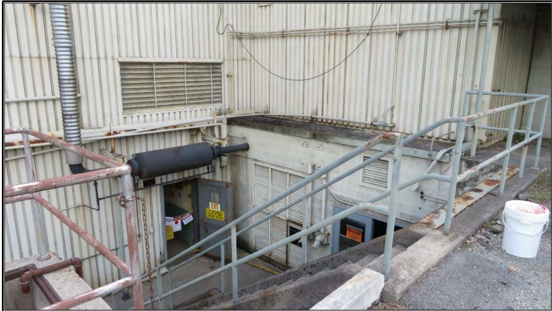
Figure A-9. Current photograph showing the retaining wall enclosed well on the north elevation of Building 3042, providing access to the below-grade first floor, facing southwest.
