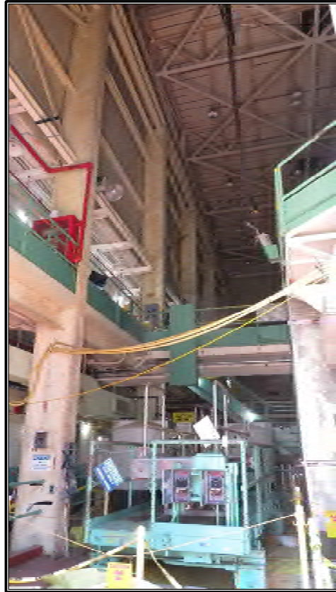
Figure A-17. Current photograph showing the north portion of the high bay in Building 3042 as seen from the second-level service entry on the west elevation, facing east.
