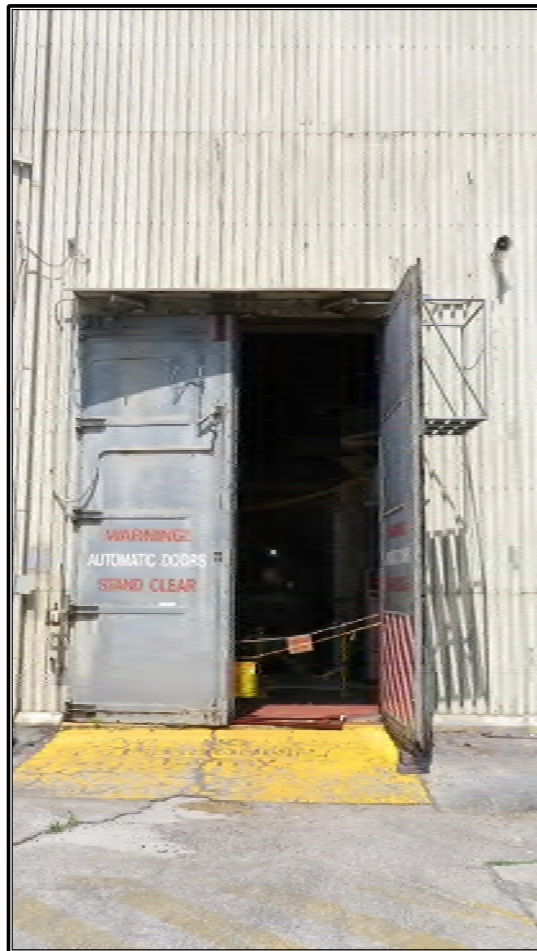
Figure A-6. Current photograph showing the service entry on the west elevation of Building 3042, facing east.
