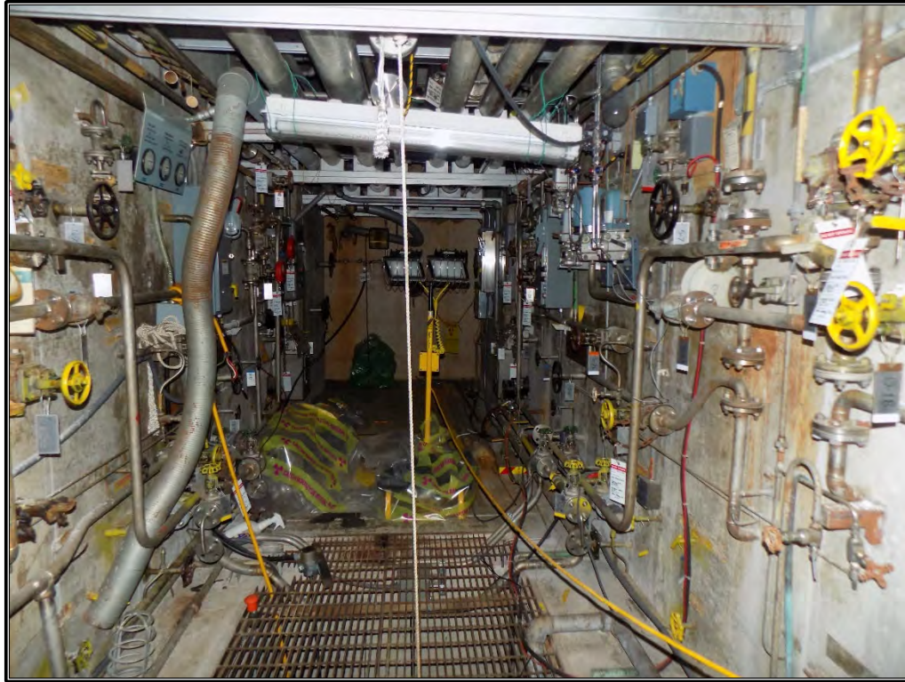
Figure A-11. Current photograph showing the ORR pipe corridor, or pipe chase, in the basement of Building 3042.
