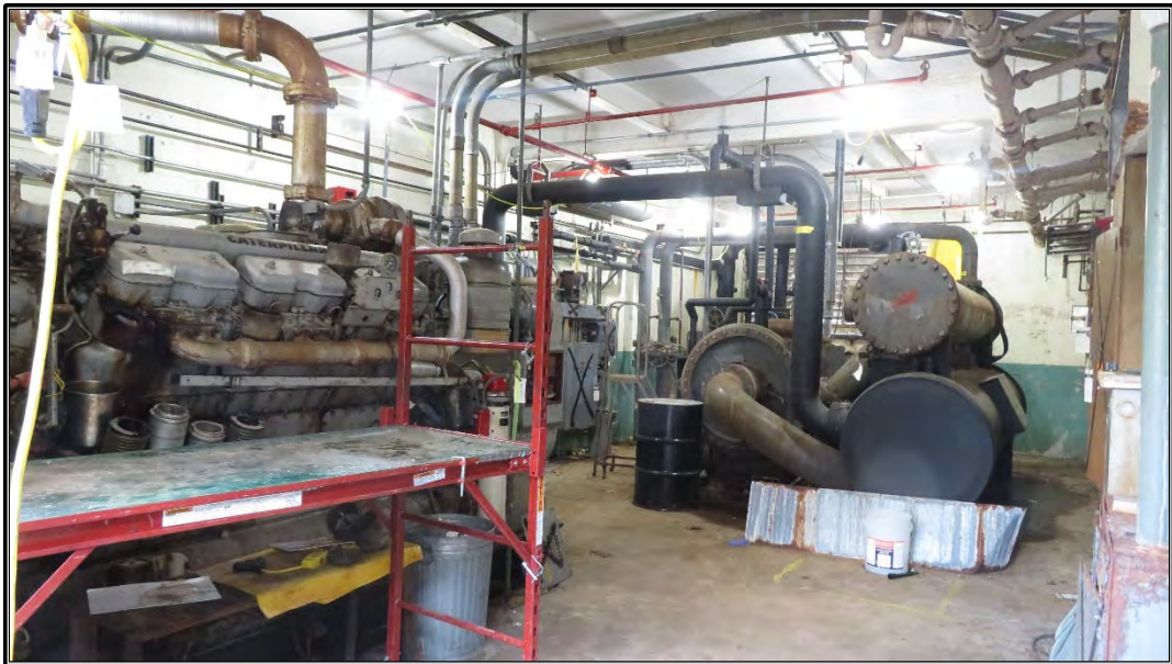
Figure A-22. Current photograph showing the Equipment Room, located on the first floor of the circa 1957 Change Room addition on the north elevation of Building 3042, facing west.
