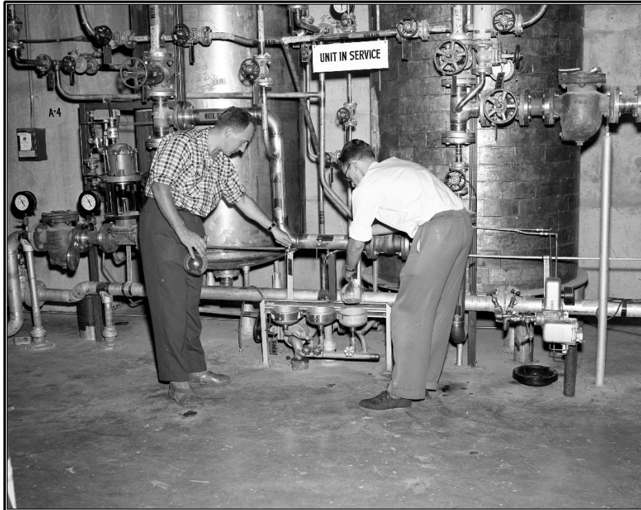
Figure A-47. Archival photograph showing employees working with the anion and cation exchangers located on the west wall in the basement of Building 3042, circa 1959 (ORNL Photo 47539).
