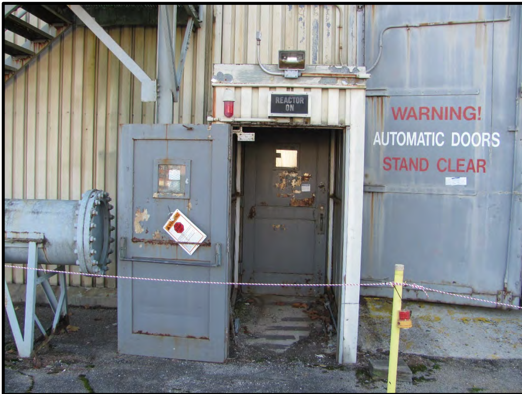
Figure A-2. Current photograph showing the vestibule on the east elevation of Building 3042, facing west.
