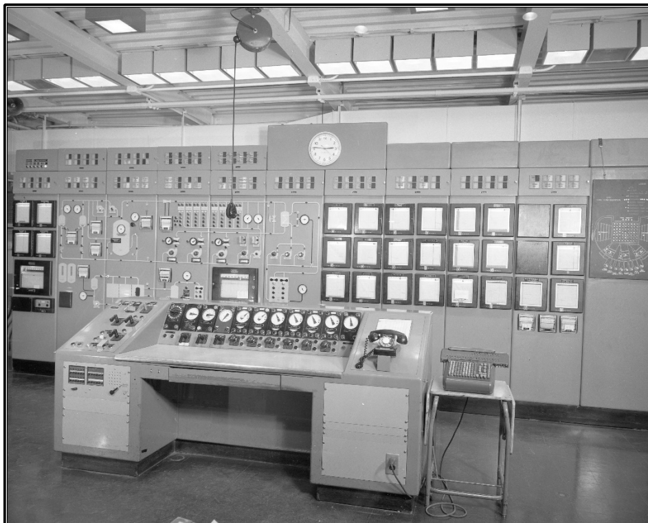
Figure A-60. Archival photograph of the Control Room on the third floor of the north wing in Building 3042, facing north, circa 1962 (ORNL Photo 59471).
