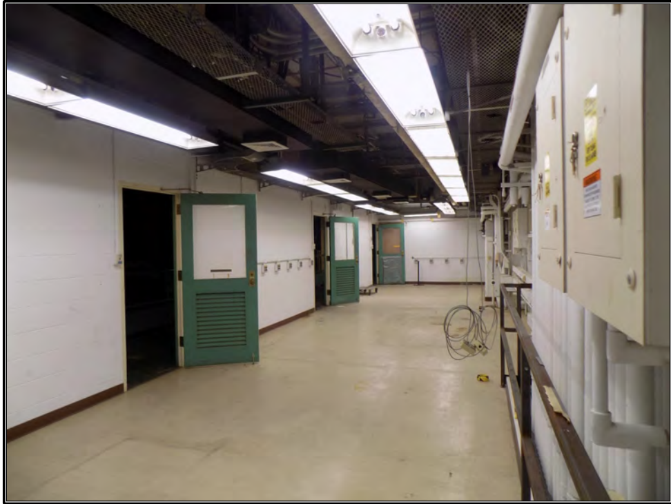
Figure 110. Current photograph showing the Control Room for in-pile experiments, facing southwest.
