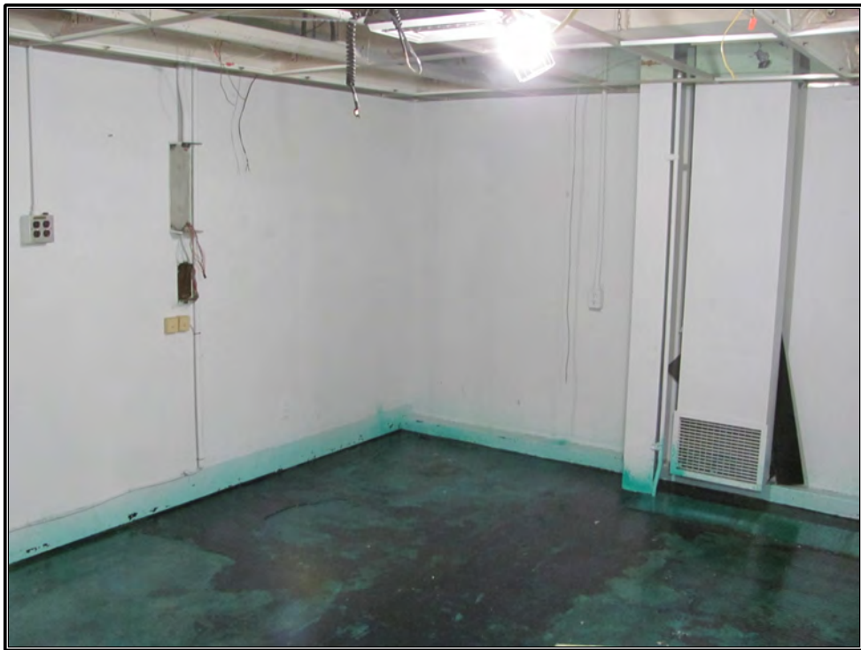
Figure 127. Current photograph showing an example of an office on the third floor of the south wing in Building 3042.
