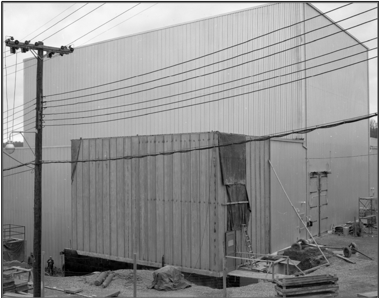
Figure 25. Archival photograph of change house extension on the north elevation of Building 3042, circa 1957 (ORNL Photo 42104).
