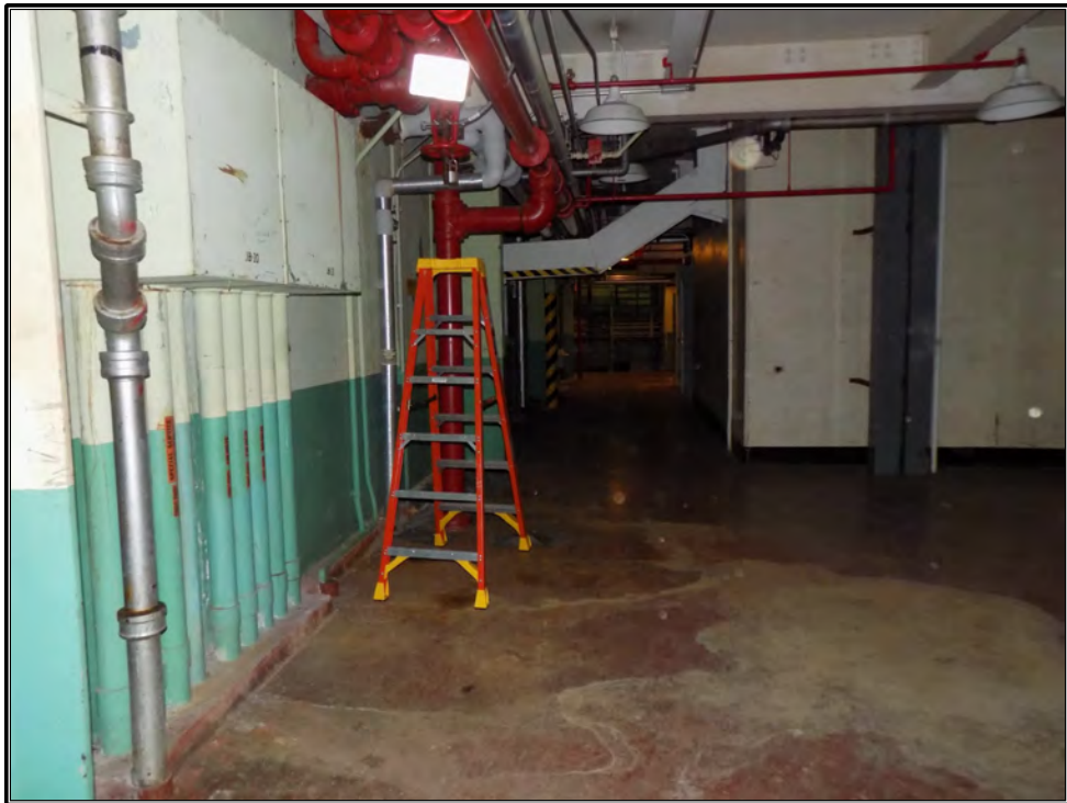
Figure 101. Current photograph showing the corridor between the reactor structure and the west wall of the first floor in Building 3042, facing north.
