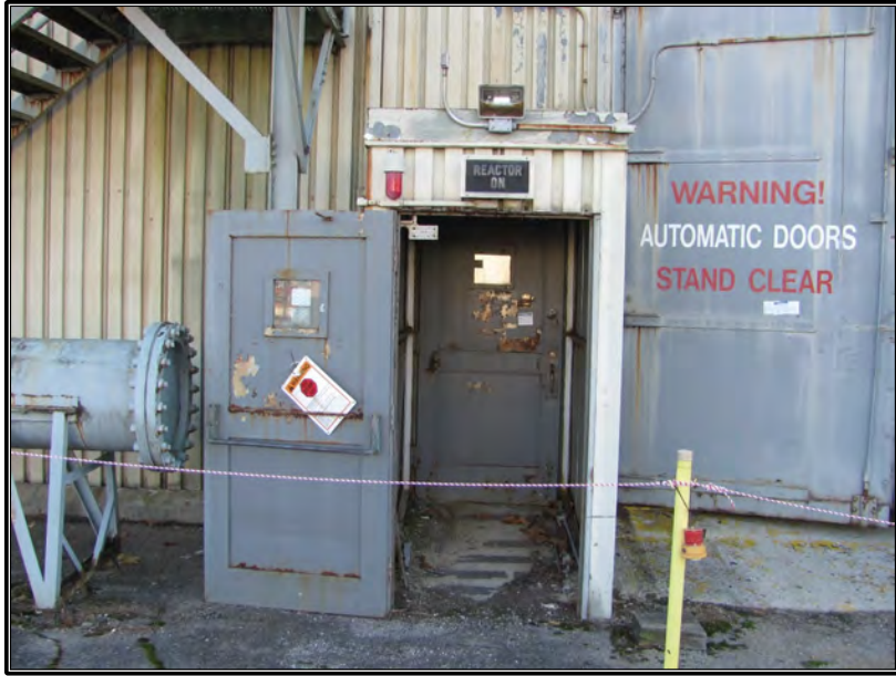
Figure 43. Current photograph of vestibule south of the service entry on the east elevation of Building 3042, facing west.
