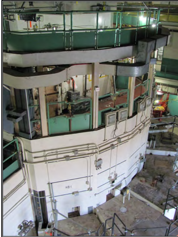
Figure 9. Current photograph of the reactor facility in the high-bay section of Building 3042, facing northwest.
