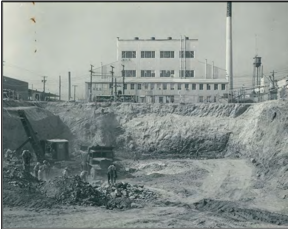
Figure 14. Archival photograph of the construction of Building 3042 showing the initial excavation of the site, September 23, 1955 (ORNL Photo 55-0836).
