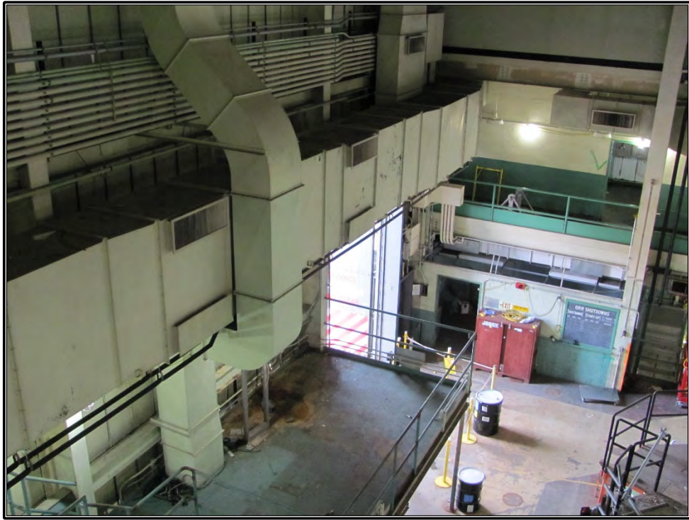
Figure 131. Current photograph showing the east portion of the third floor in Building 3042, facing southeast.
