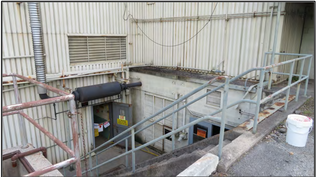
Figure 59. Current photograph of north elevation of Building 3042 showing concrete-lined well with two below-grade entries.
