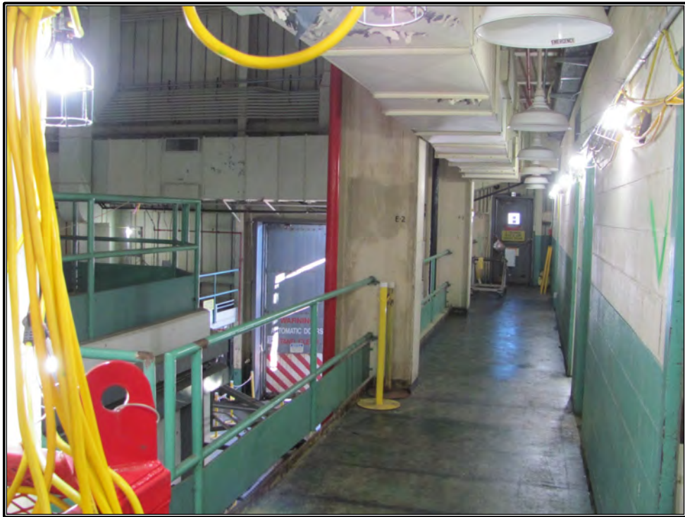
Figure 119. Current photograph of the east end of the south corridor, facing northeast. At right the single-leaf entry accesses the fire escape on the east elevation; at left the service truck entry accesses the first floor of Building 3042 from the east elevation.
