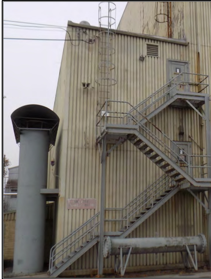
Figure 45. Current photograph of east elevation of south wing of Building 3042, facing west.
