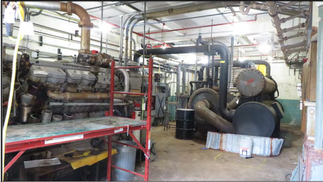
Figure 103. Current photograph of first floor of the northwest addition to Building 3042, looking south. At right is a compressor; at left is a generator.
