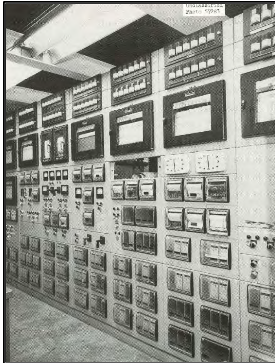
Figure 220. Archival photograph, circa 1964, showing the main instrument control panel for the GCR-ORR Loop No. 2 in the basement of Building 3042 (ORNL Photo 57283) (Trauger 1964:56).
