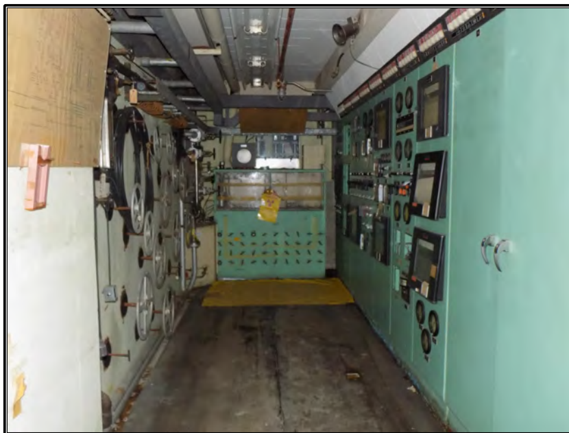
Figure 80. Current photograph showing valve extension handles for the pressurized-water loop (left), the sample station (center), and a control panel located in the Irradiation Engineering Room in the northeast corner of the basement of Building 3042, facing north.
