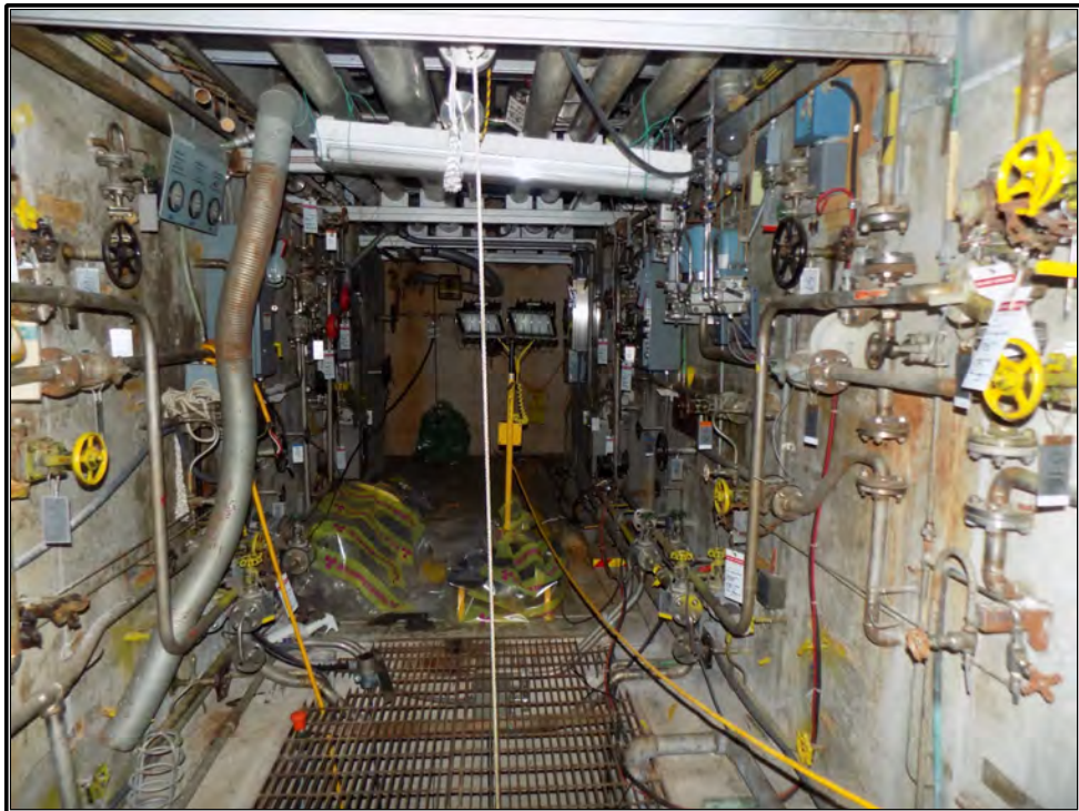
Figure 65. Current photograph showing the pipe corridor, or pipe chase, within the reactor substructure in the basement of Building 3042.
