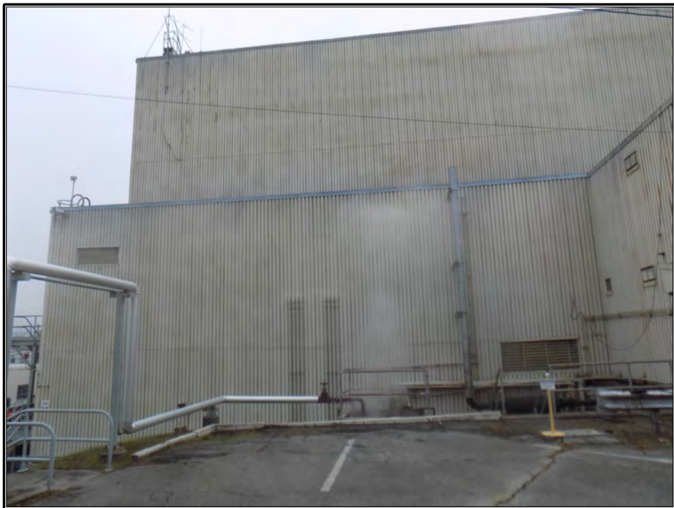
Figure 57. Current photograph of east end of north elevation of Building 3042, facing south. At right is the Change House addition constructed circa 1957; to the left of the addition is a set of stairs leading down to the first-floor level.
