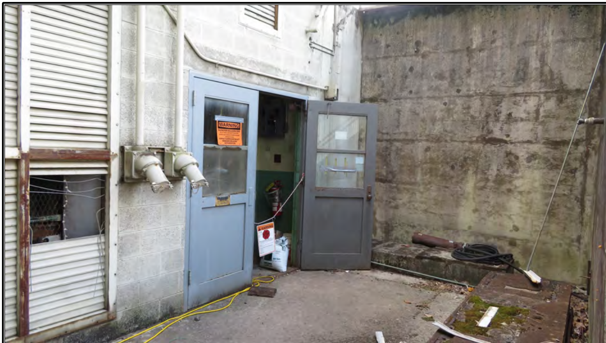
Figure 60. Current photograph of north elevation of Building 3042, facing northwest, showing the double-leaf entry in the below-grade level of the Change House addition constructed circa 1957.
