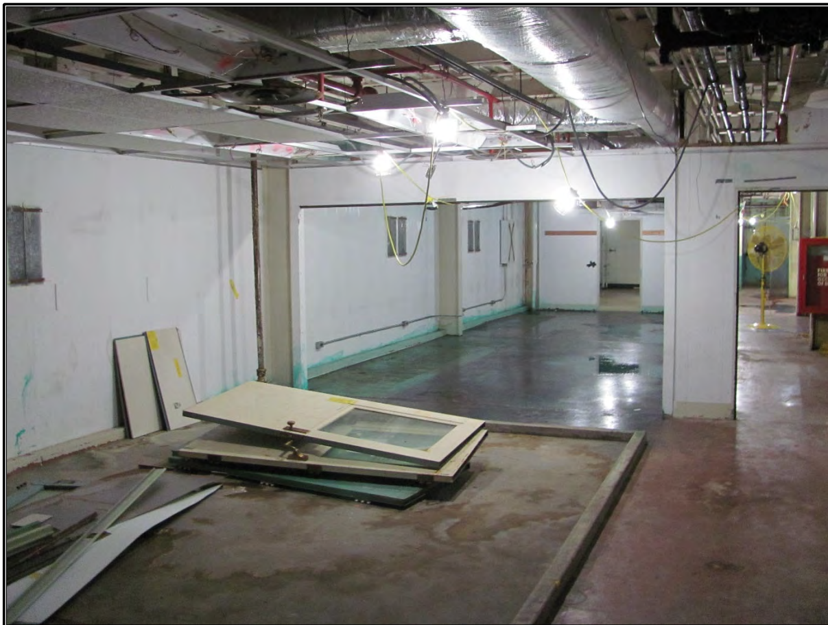
Figure 133. Current photograph showing Room 308 on the third floor of the south wing in Building 3042, facing southwest. At right the single-leaf entry accesses the third-floor south corridor.
