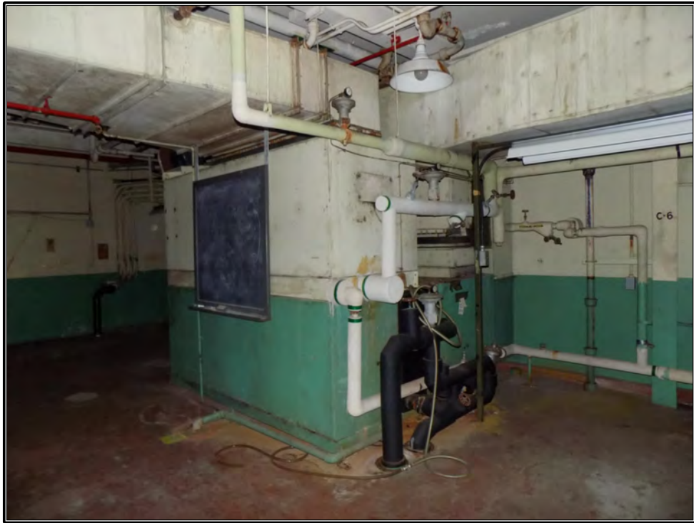
Figure 72. Current photograph showing an air-conditioning unit in the southeast corner of the basement of Building 3042, facing southeast.
