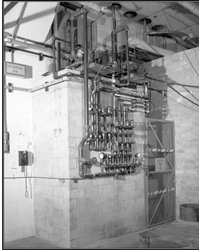
Figure 66. Archival photograph showing the southwest corner of the ORR substructure in the basement of Building 3042, including control valves mounted to the concrete block, circa 1960 (ORNL Photo 52496).
