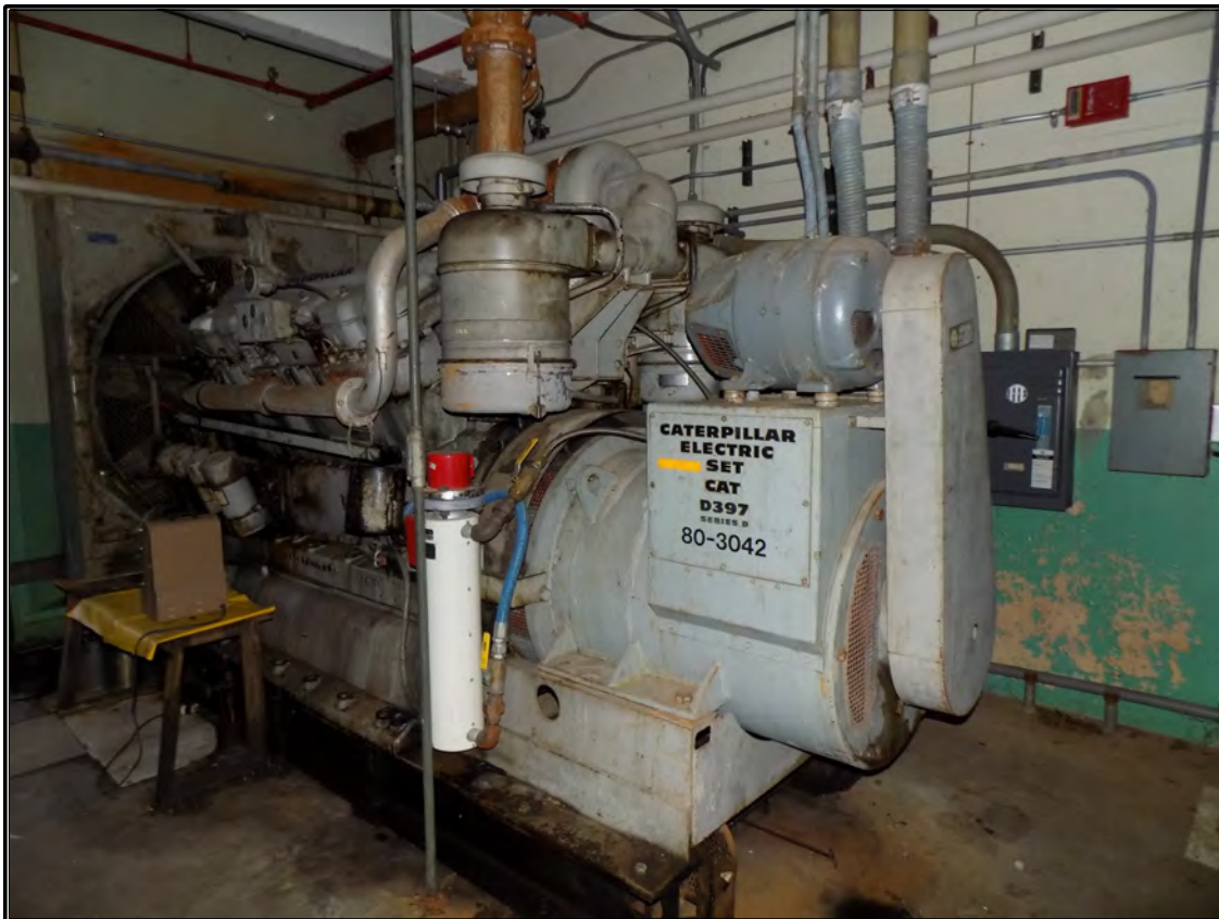
Figure 104. Current photograph showing the diesel-powered generator and box-shaped fan on the first floor of the Change House addition to Building 3042, facing southeast.
