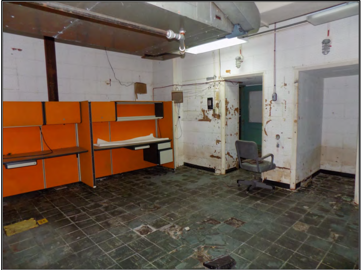
Figure 76. Current photograph of the Counting Room on the north side of the basement in Building 3042, looking southwest.
