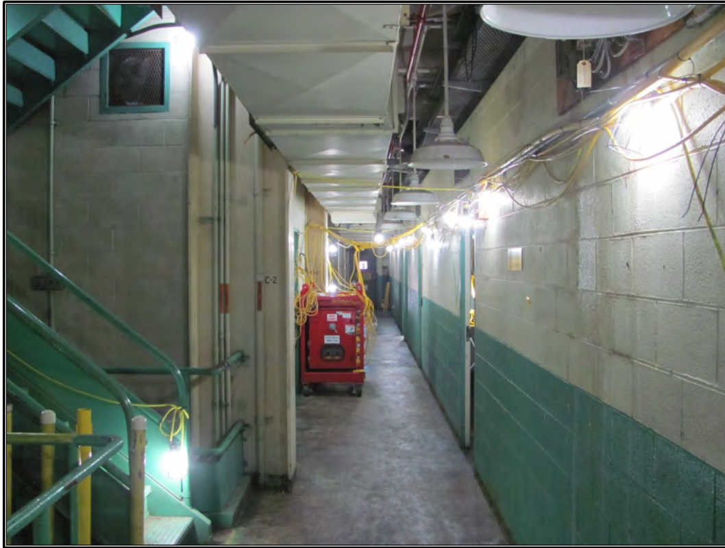
Figure 114. Current photograph of the south corridor on the second floor of Building 3042, facing east.
