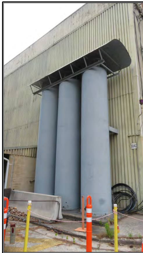
Figure 48. Current photograph of south elevation of Building 3042 showing row of tanks at southeast corner, facing northwest.
