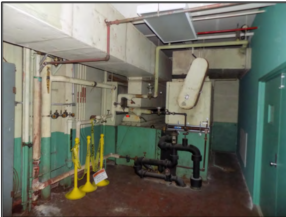
Figure 99. Current photograph showing the enclosed space in the south wing containing a large air-conditioning unit, facing west.
