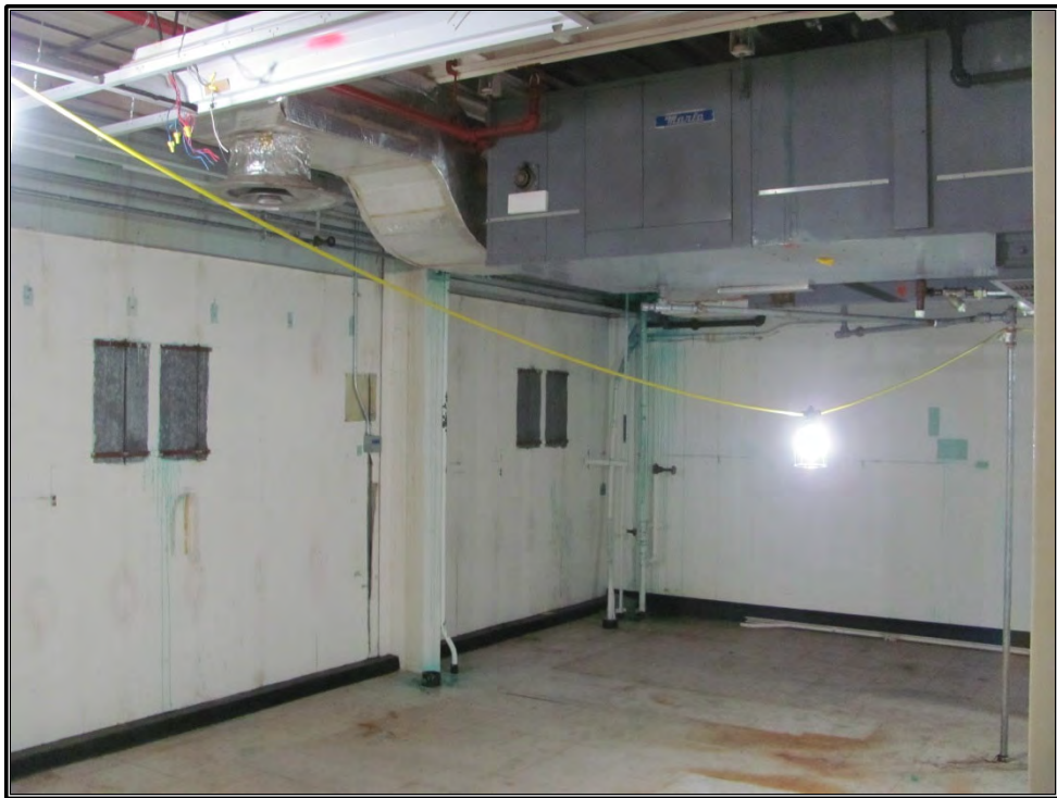
Figure 132. Current photograph showing Room 302 in the south wing of the third floor of Building 3042.
