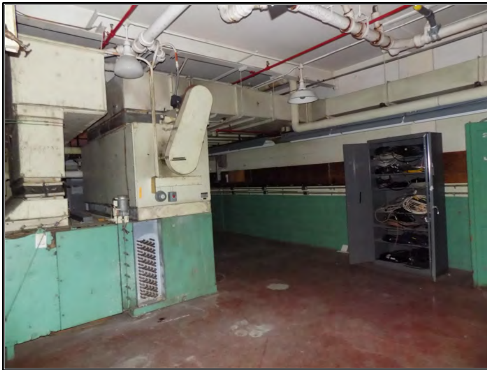
Figure 88. Current photograph of Instrument Staff Shop area on the north side of the first floor of Building 3042. At left is the air-conditioning unit shown in the previous figure.
