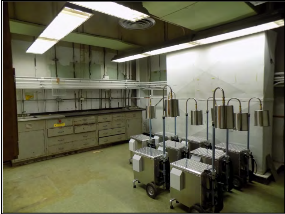
Figure 118. Current photograph of the Reactor Maintenance Plant and Equipment Division Office in the southeast corner of the second floor of Building 3042, facing southeast.
