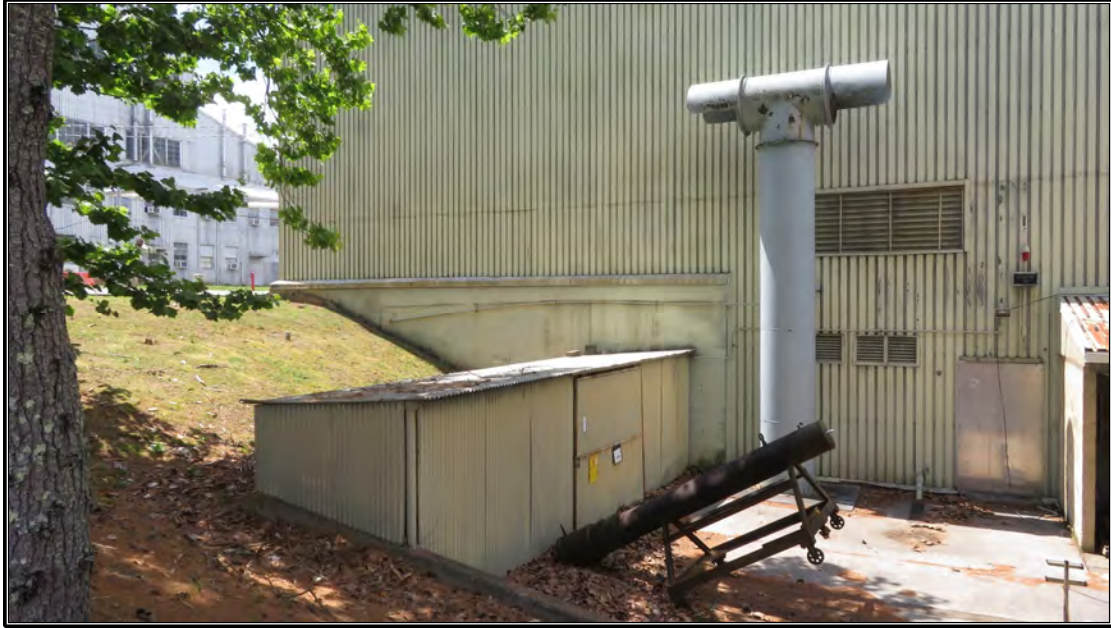
Figure 49. Current photograph of south elevation of Building 3042 showing the metal-panel addition, facing north.
