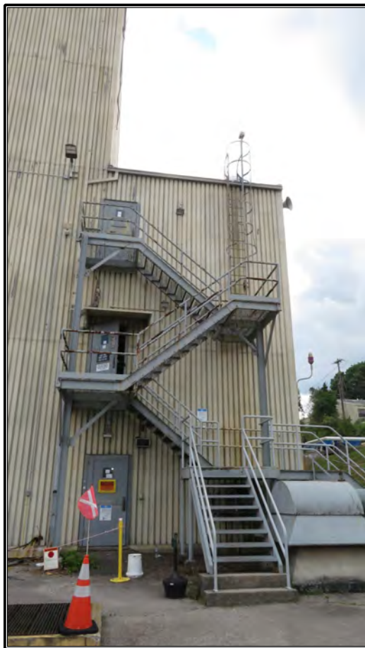
Figure 44. Current photograph of east elevation of north wing of Building 3042, facing west.
