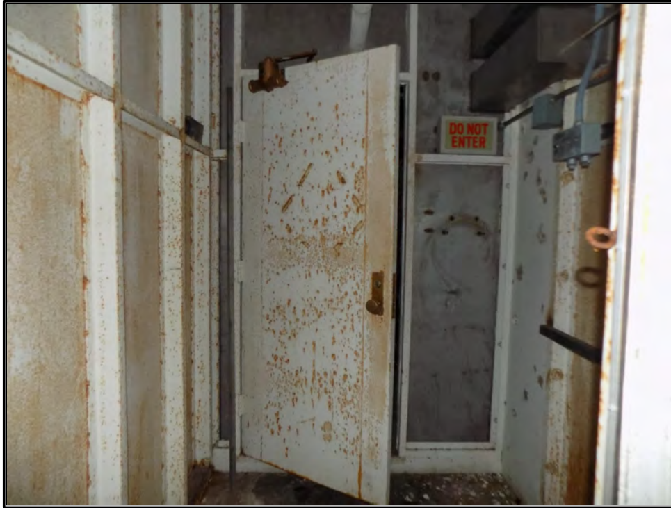
Figure 96. Current photograph showing the Air Lock providing access to the Decontamination Room which provides access to the interior of the containment cell on the south side of the reactor structure, facing north.
