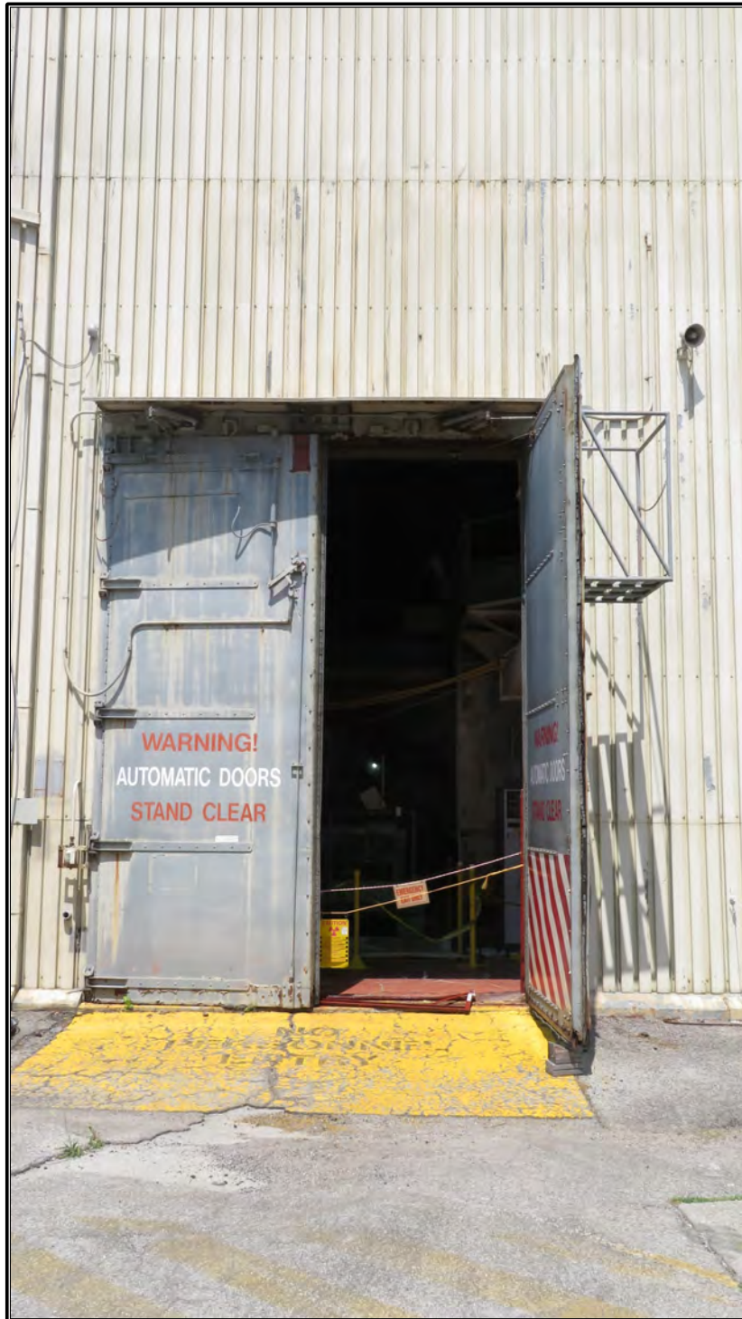
Figure 54. Current photograph of service entry on the west elevation of Building 3042, facing east.
