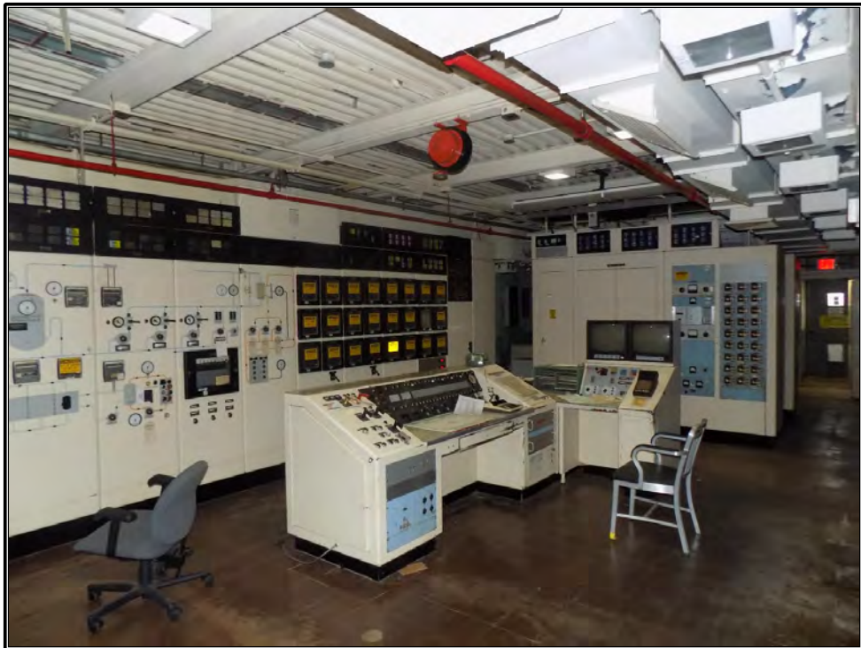
Figure 130. Current photograph showing the Control Room, or Room 309, in the third-floor north wing of Building 3042, facing northeast. At right, the single-leaf entry leads to the northern fire escape on the east elevation.
