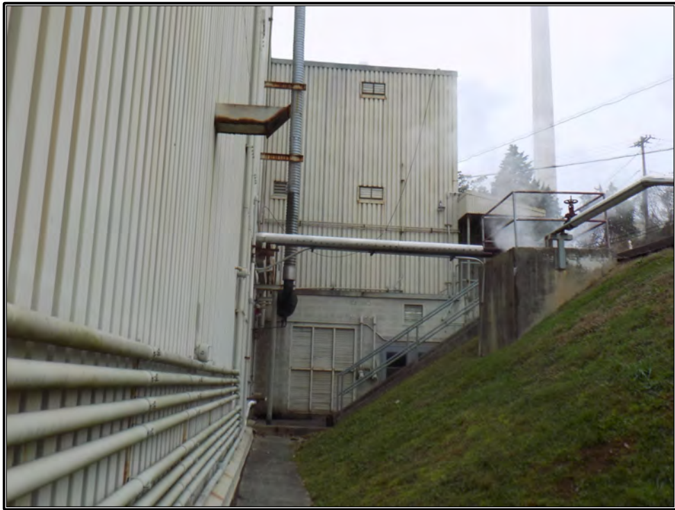
Figure 58. Current photograph of north side of Building 3042, facing west toward the Change House addition constructed circa 1957.
