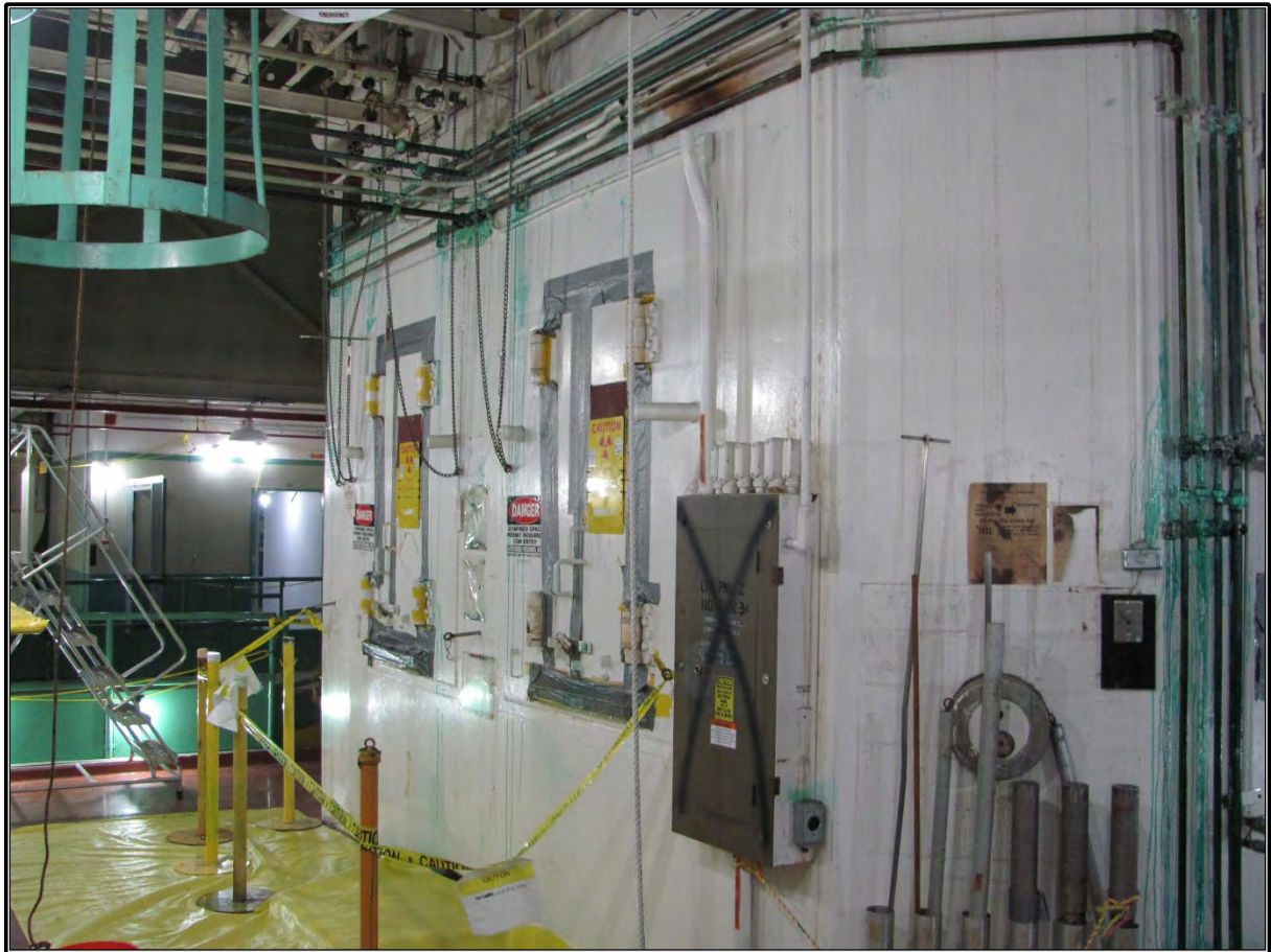
Figure 136. Current photograph showing the west elevation of the hot cell structure located at the west end of the reactor structure in Building 3042, facing northeast.
