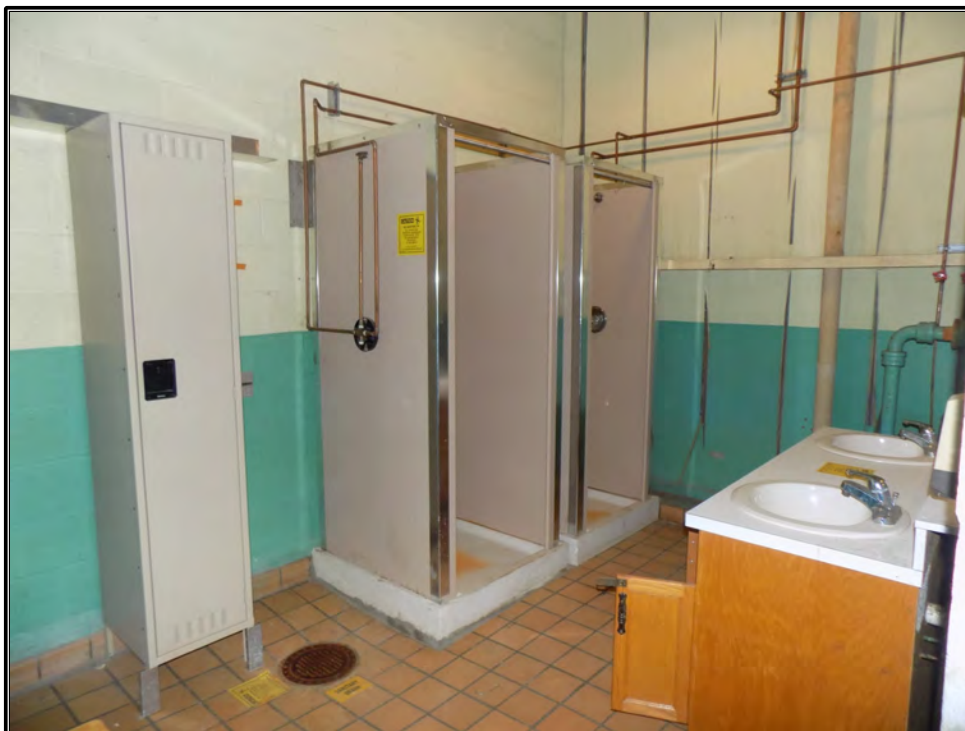
Figure 107. Current photograph of women's restroom in the northwest portion of the south wing on the second floor of Building 3042, showing locker area and showers.
