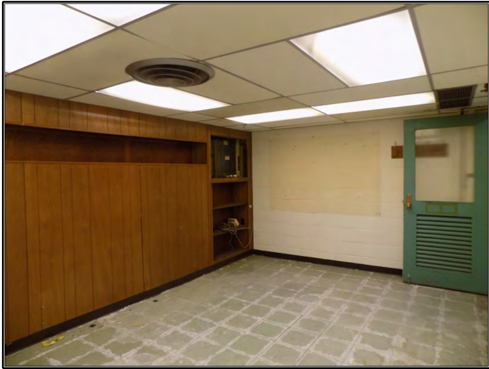
Figure 116. Current photograph showing Room 204 on the second floor of the south wing in Building 3042, facing southwest.
