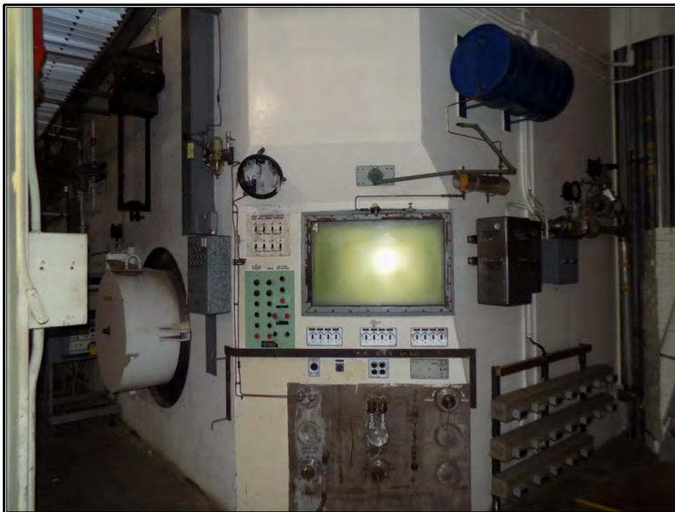
Figure 95. Current photograph showing the southeast corner of the containment cell on the south side of the reactor structure, facing northwest. At left, a metal plug shields the access to a large port piercing the south wall of the containment cell.
