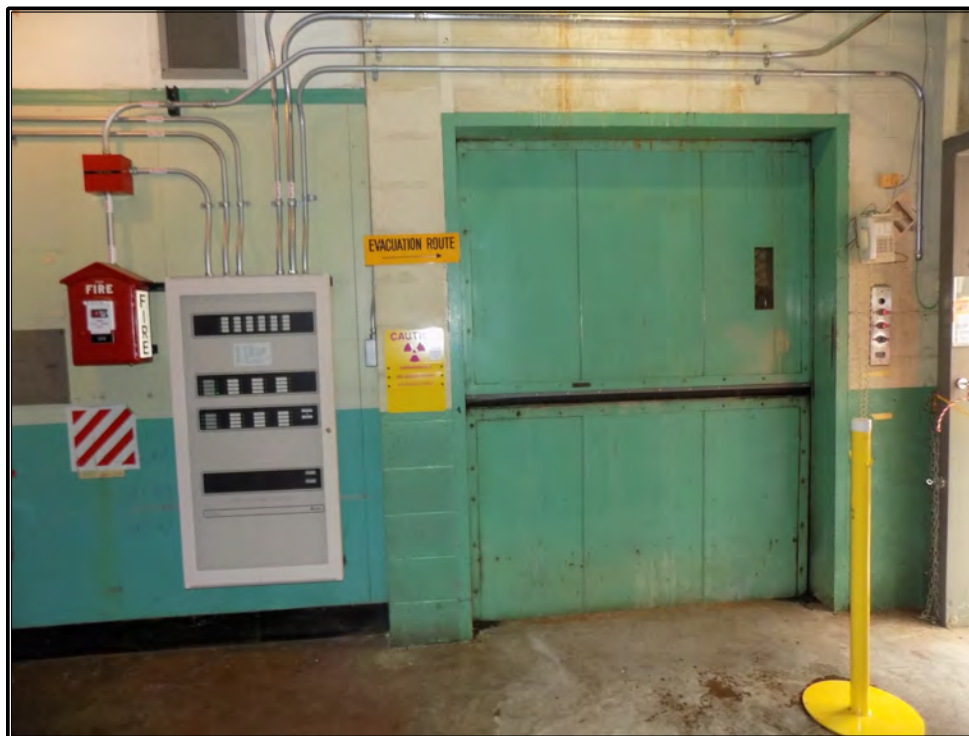
Figure 115. Current photograph showing the elevator door in the southwest corner of the second floor of Building 3042, facing south.
