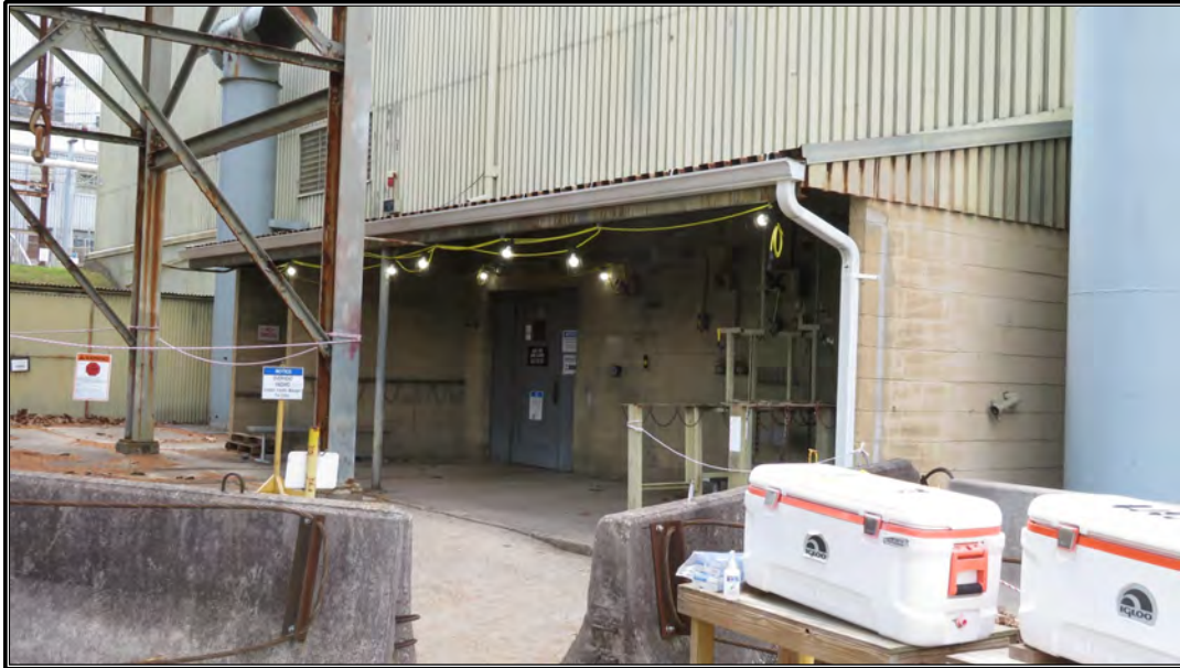
Figure 47. Current photograph of south elevation of Building 3042 showing concrete-block addition, facing northwest.
