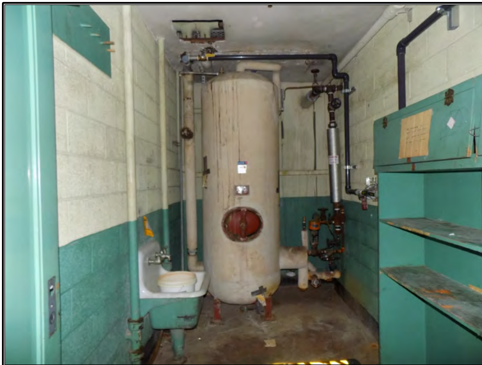
Figure 109. Current photograph of janitor's closet with hot water heater, located in the northwest corner of the second floor of Building 3042, facing south.
