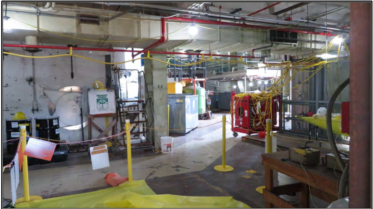
Figure 93. Current photograph showing the south side of the first floor and reactor structure in Building 3042, facing northeast.
