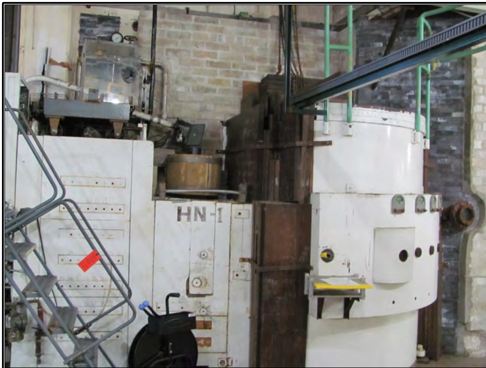
Figure 92. Current photograph showing the North Engineering Test Facility equipment located on the north side of the reactor structure, facing southwest.
