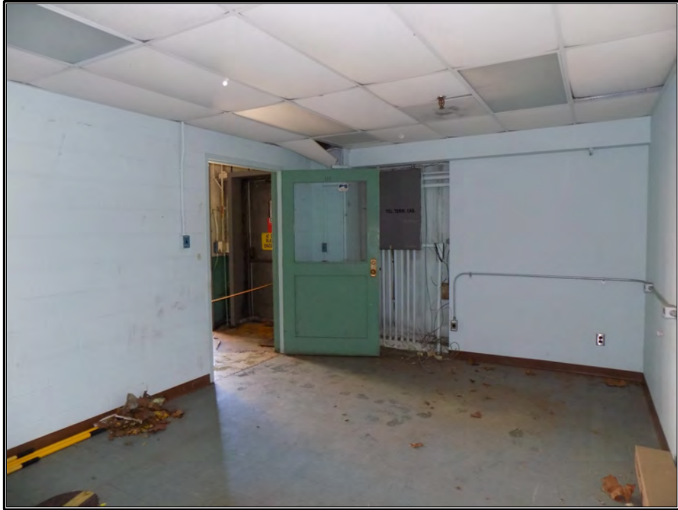
Figure 100. Current photograph showing the room occupying the southeast corner of the first floor of Building 3042, facing northeast.
