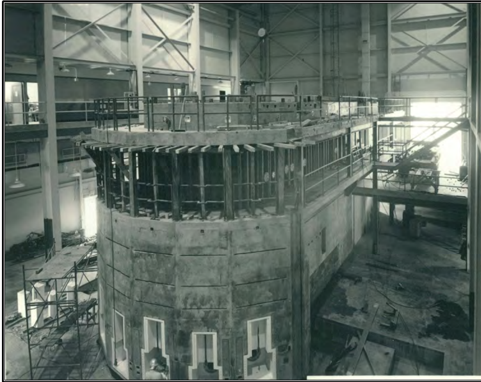
Figure 20. Archival photograph of the construction of Building 3042 showing the ORR structure in the high bay, April 18, 1957; along the bottom of the structure are six beam holes for use in experiments (ORNL Photo 57-0510).
