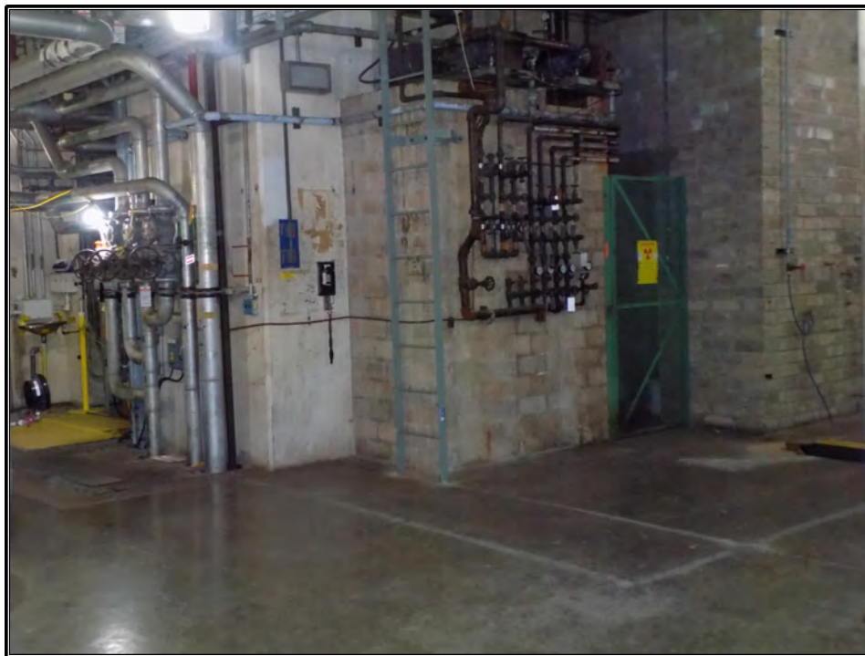
Figure 67. Current photograph showing the southwest corner of the ORR substructure in the basement of Building 3042, facing northeast.
