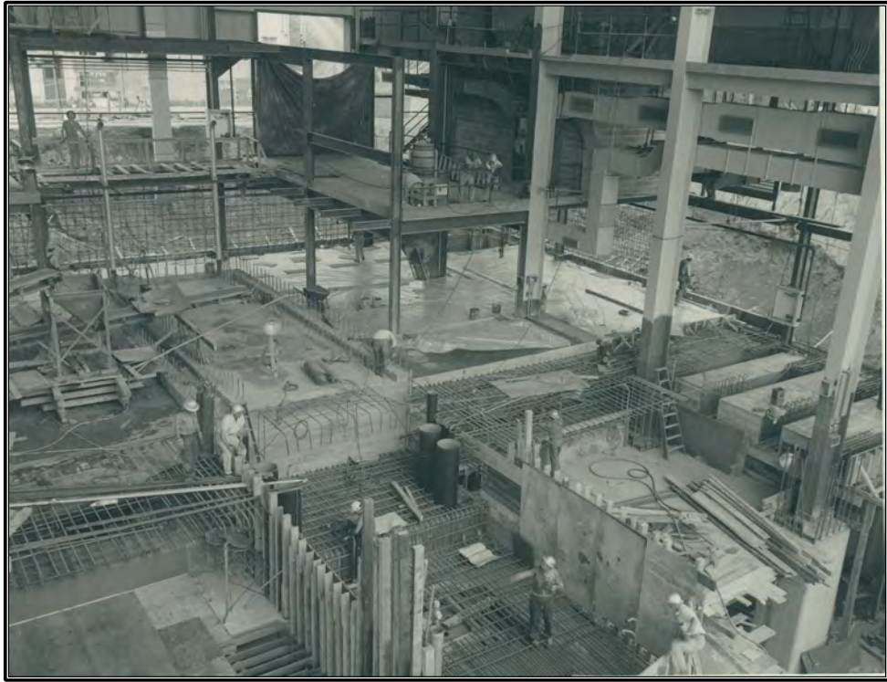
Figure 18. Archival photograph of the construction of Building 3042 showing the interior looking toward the west wall, July 18, 1956 (ORNL Photo 56-0715).
