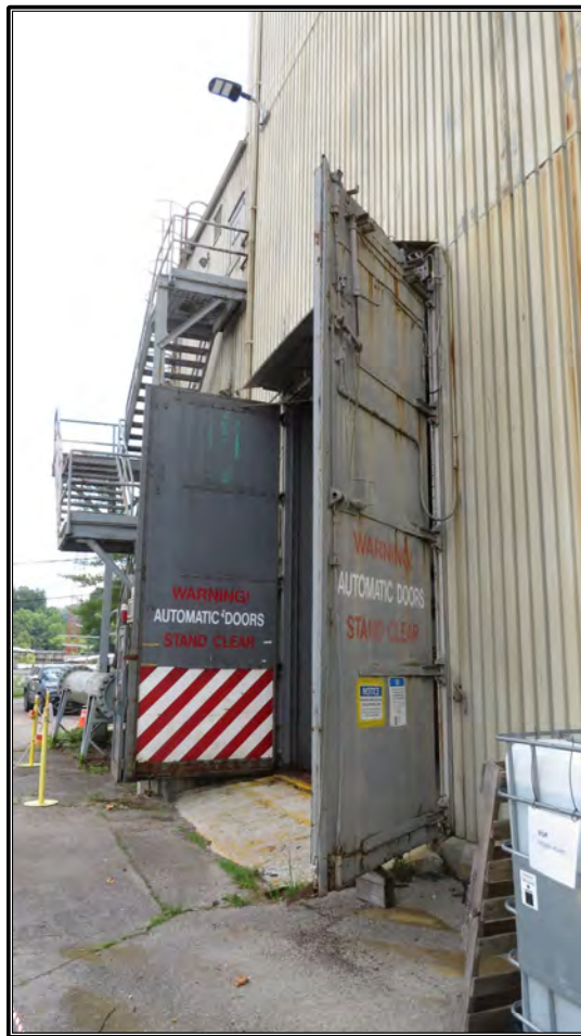
Figure 42. Current photograph of service entry on the east elevation of Building 3042, facing south.
