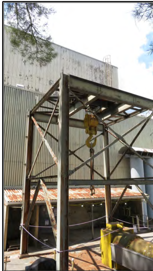
Figure 50. Current photograph showing gantry and crane adjacent to the south elevation of Building 3042, facing north. The south elevation of the high-bay appears at top.
