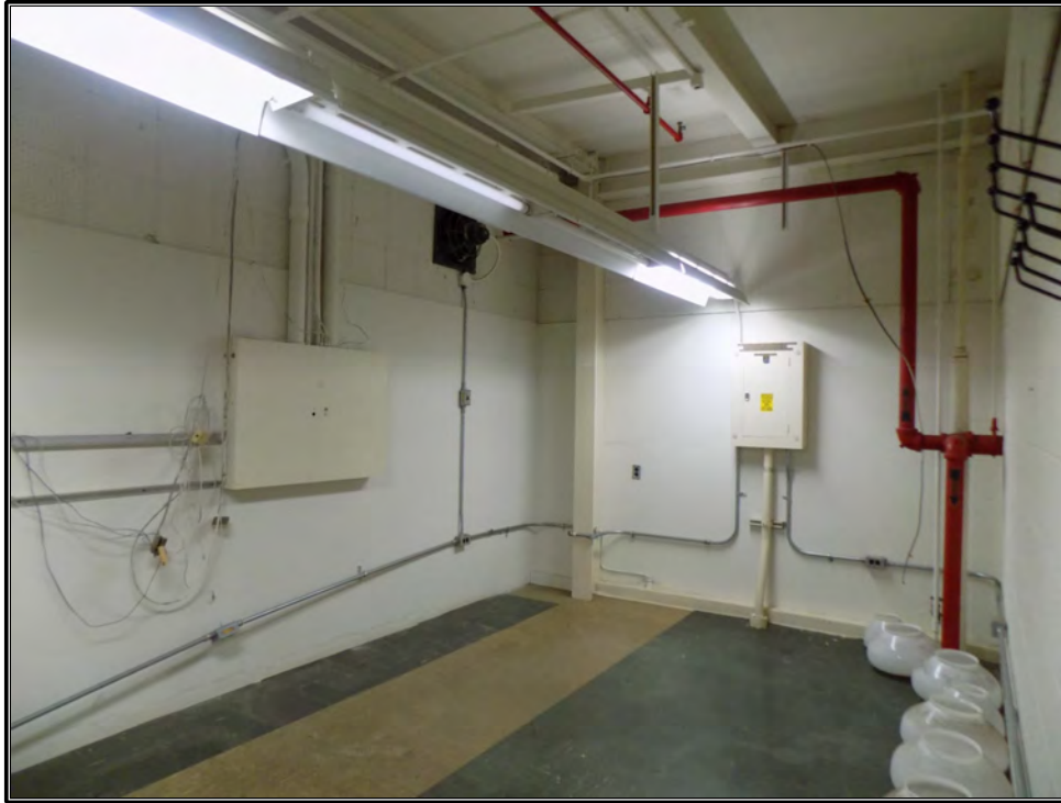
Figure 98. Current photograph showing the Instrumentation Room on the first floor of Building 3042, facing southeast.
