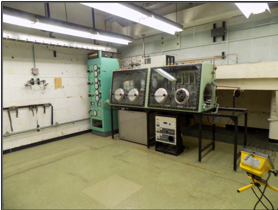
Figure 113. Current photograph showing Room 212 located along the south side of the reactor structure at the second-floor level of Building 3042, facing northwest.
