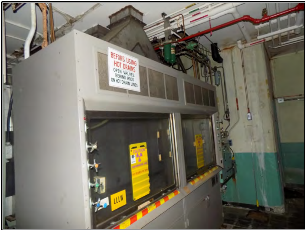
Figure 75. Current photograph of a fume hood in the Laboratory on the north side of the basement in Building 3042.
