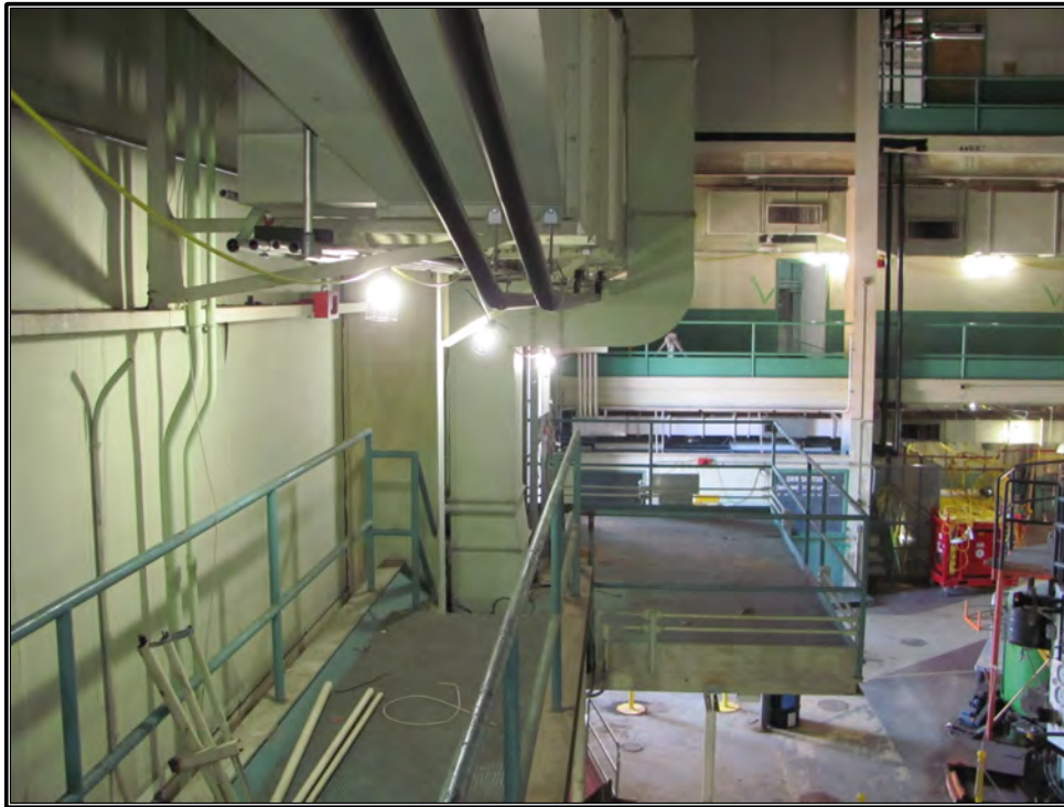
Figure 112. Current photograph showing the catwalk (at left) and the suspended platform (at center) on the east wall of Building 3042 at the second-floor level, taken from the east end of the north corridor, facing south.
