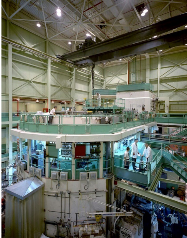
Fig. 3. The Bldg. 3042 high bay, circa 1967, showing the ORR with its four working levels for research and isotope production.
