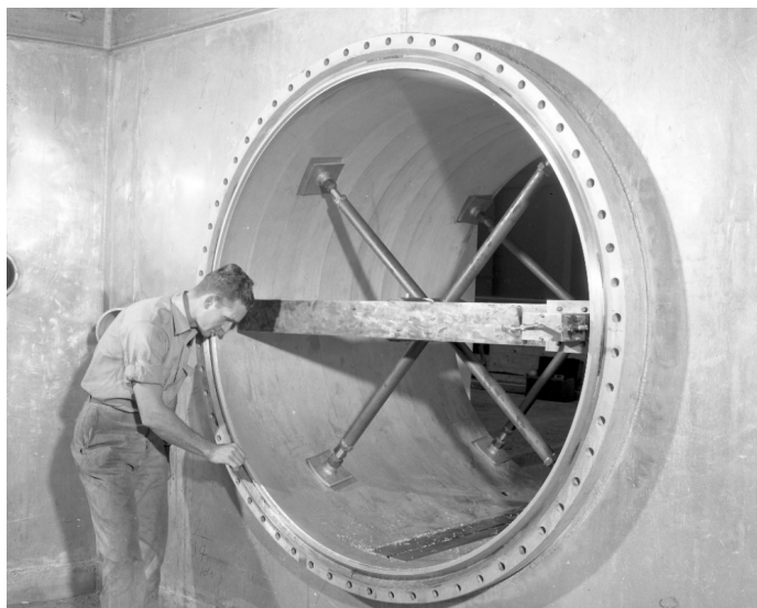
Fig. 5. The exterior of one of the ORR large engineering test facilities while under construction, circa 1957.
