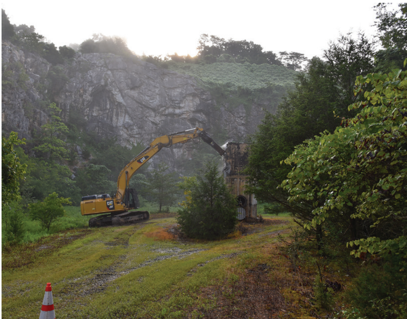
Demolition of the K-1099 seismic instrument facility at Blair Quarry, one of several small structures removed during the fiscal year
