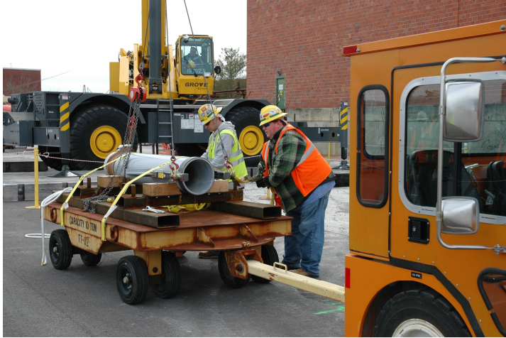
NaF trap practice: Workers practice lifting a dummy NaF trap as part of preparation for the actual job. Pictured are crane operator Chester Sheldon, and riggers Michael Shirks (left) and Larry Leonard.
