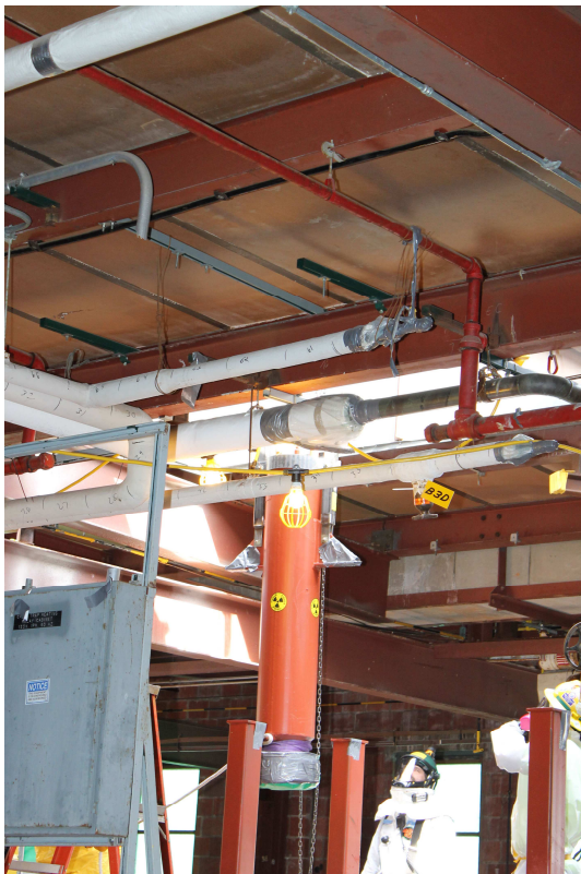
NaF trap being removed: Ernie Gunter (left) and Michael Shirks watch as a NaF trip is lifted through the roof of K-27.
