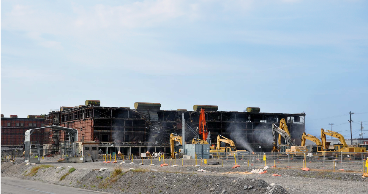
Workers began demolishing the remaining section of the K-25 building today (Sept. 17).
