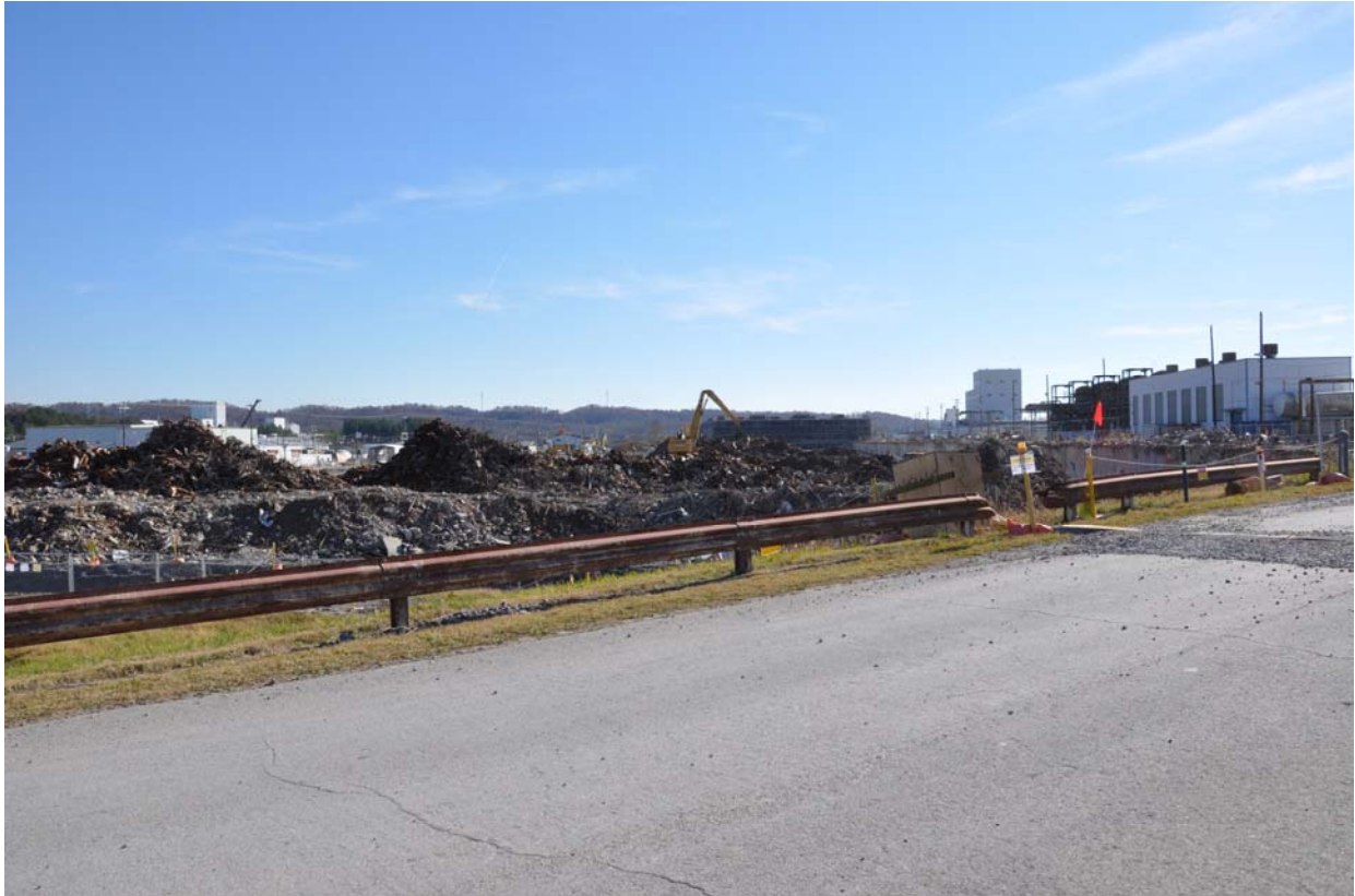
Cutline for Photo: Some of the debris from the demolition of K-25's east wing.
