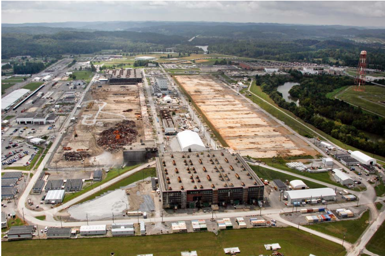
Caption: Workers were wrapping up the east wing demolition when this photo was taken on Sept. 5. The north end sits in the foreground.
