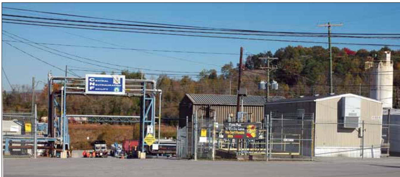
Central Neutralization Facility
