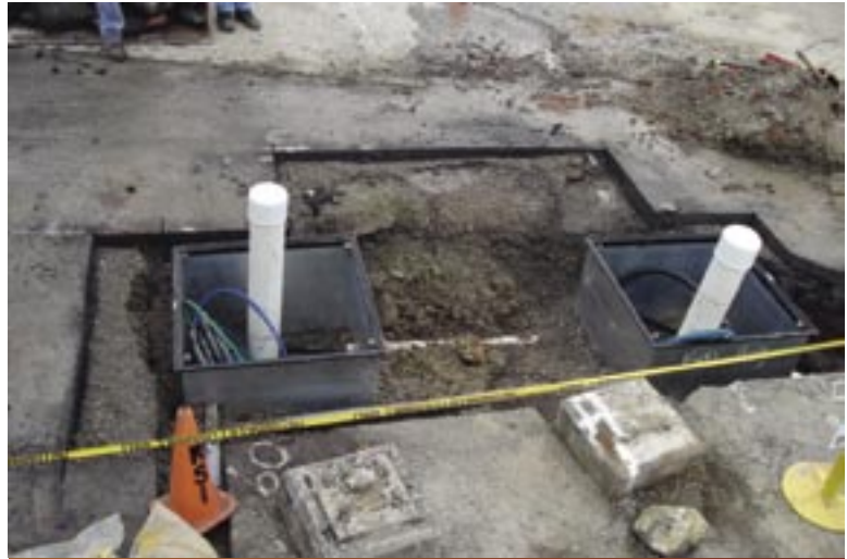
Installation of the water treatment system for hexavalent chromium at Mitchell Branch
