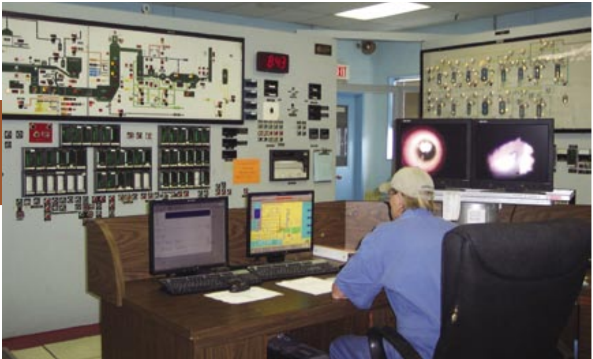
TSCA Control Room
