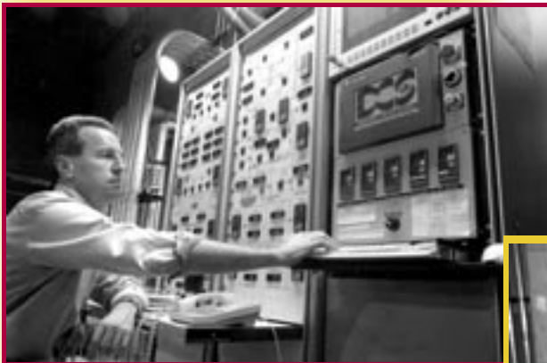
MSRE process control panels
