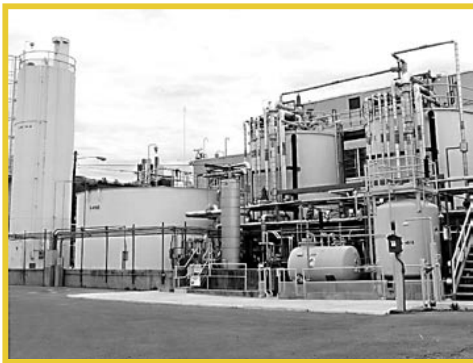
More than 35 million gallons of waste were treated at the Central Neutralization Facility in FY 2003
